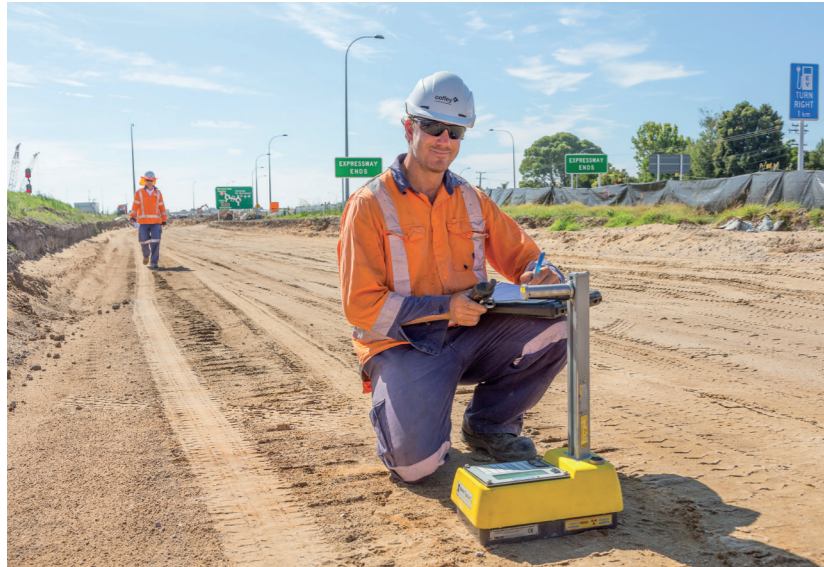
Earthworks compaction testing is carried out on what will become the new city-bound lanes near the Te Maunga roundabout. Compaction testing is required whenever any earthworks are carried out to ensure the ground has compacted sufficiently before the road is built on top.
