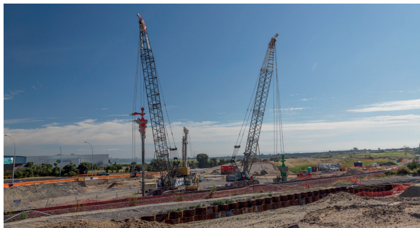
Stone column ground improvement is continuing in the Baypark area, with two cranes dedicated to the job. Stone columns involve putting vertical columns of stone (gravel) into the ground and using vibration to force stone into the sand layers and make it strong enough to support construction on top of it.
