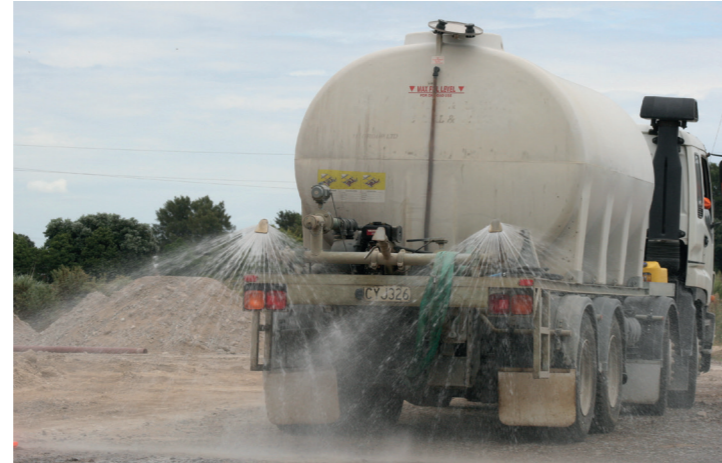
One of the water tankers used for dust management throughout the Bay Link site.
