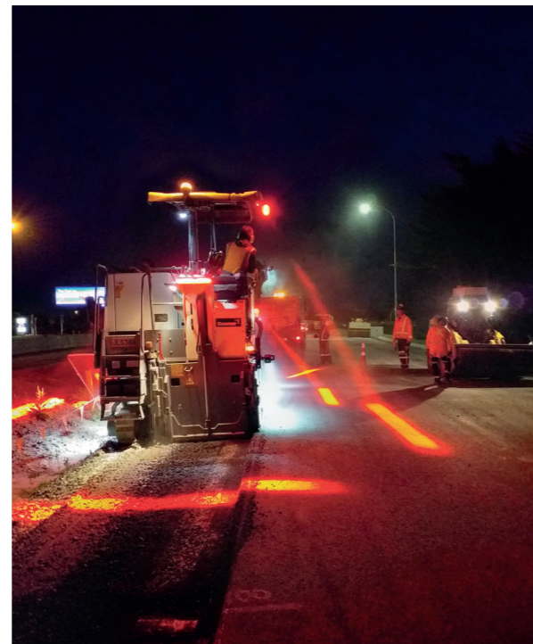
Asphalting near the existing road between Jackson Street and Concord Avenue in preparation for the traffic switch. The beams of light on the ground indicate the plant operating zone, so the team on the ground know to stay clear at all times. It's a practical and effective safety initiative for night works.
