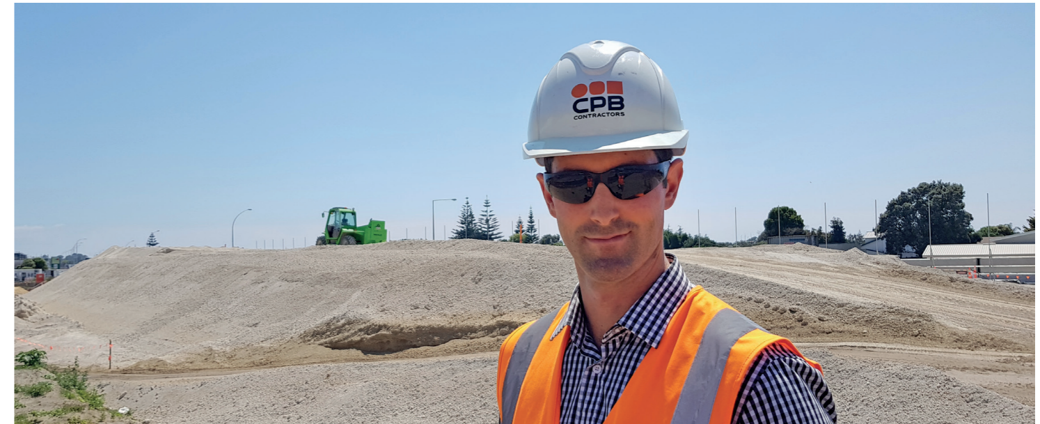
Senior Project Engineer Brad Wallace likens the ground conditions beneath the embankment to a 15m stack of pancakes.
