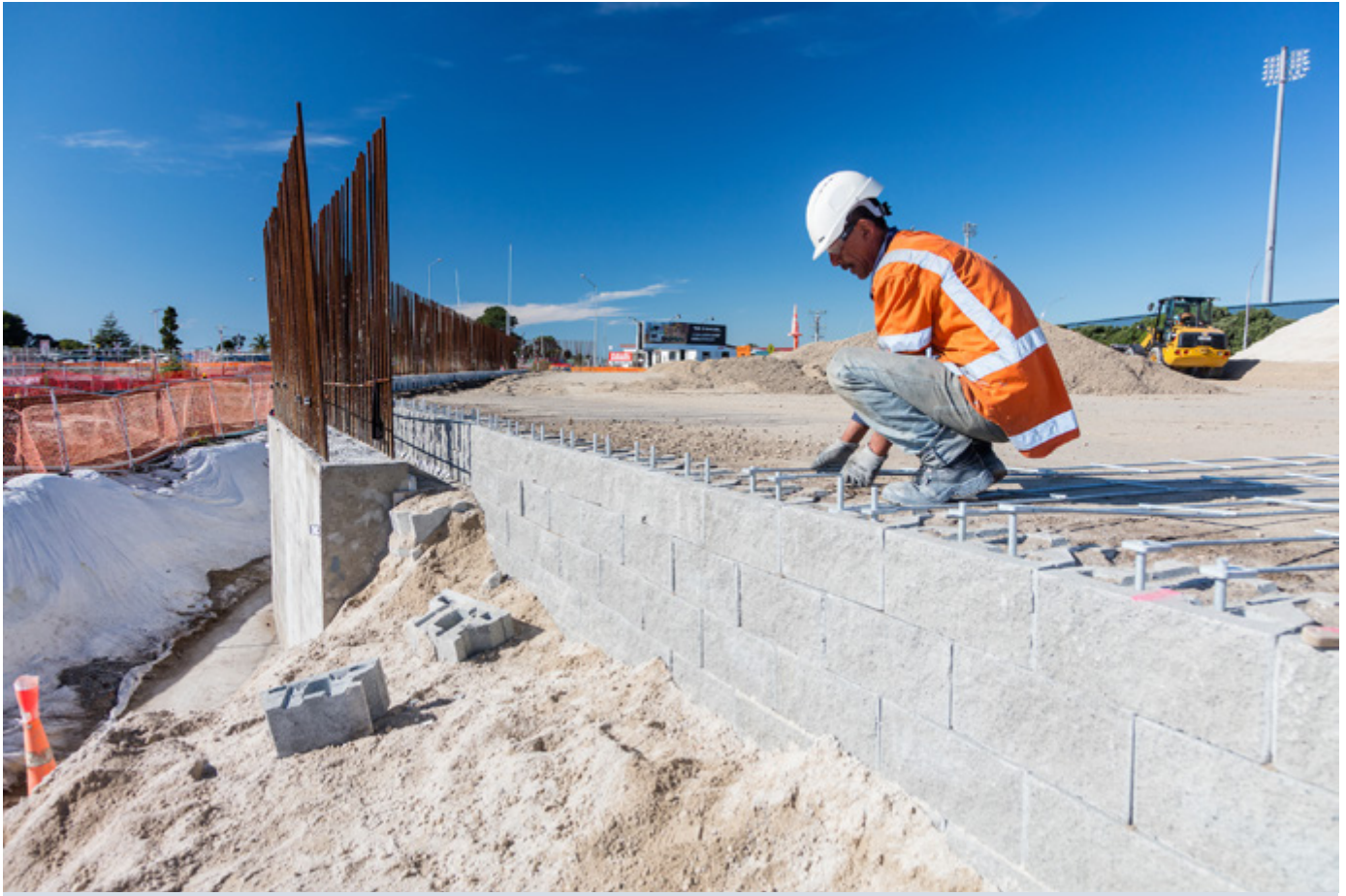
A mechanically stabilised earth wall under construction using concrete blocks and steel reinforcing ladders
