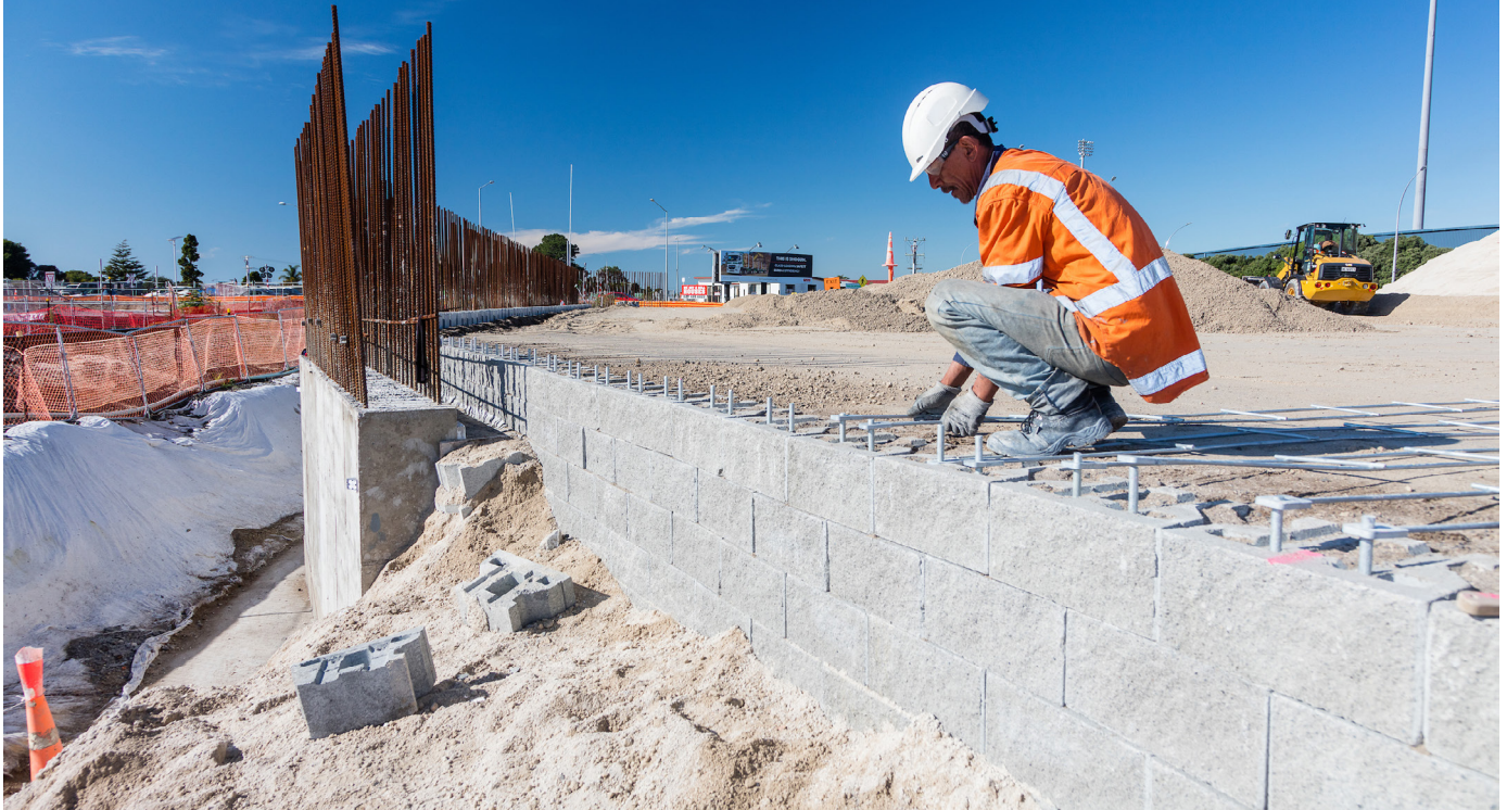
A mechanically stabilised earth wall under construction using concrete blocks and steel reinforcing ladders
