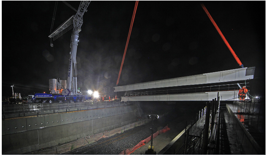
Beams being placed on the rail bridge at Te Maunga in February
