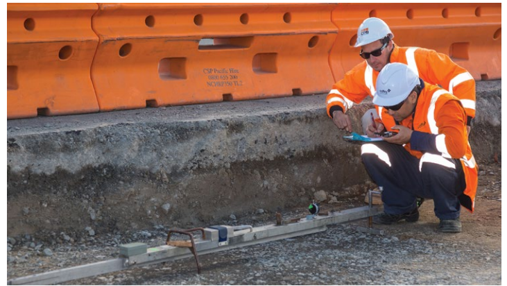
Bay Link workers use a Benkelman Beam to measure the deflection of the sub grade level on a new section of Girven Road. Deflection is the degree to which a road formation moves under a known load and helps ensure the road will meet the requirements for the traffic load that will be using it once completed.
