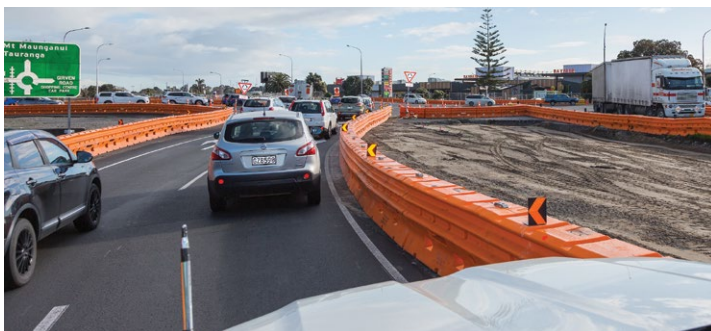
Temporary speed limits are in place throughout the Bay Link construction site for the safety of all road users and our construction workers. We thank you for your patience while we carry out the work in this area.
