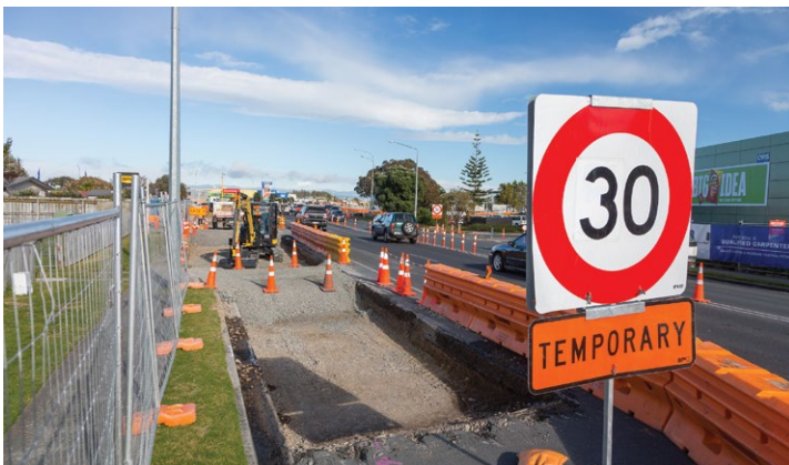
The first section of road widening work is nearing completion on Girven Road, between Gloucester Road and the Bayfair roundabout, including installation of a new water main, new concrete kerbing and footpath, and laying asphalt.
