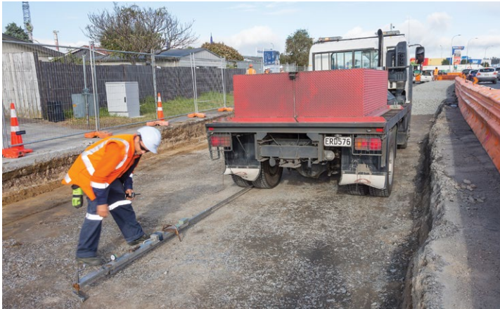
A Benkelman Beam is used behind a weighted truck on a new section of Girven Road. Measurement is made by placing the tip of the beam between the dual tyres and measuring the pavement surface rebound as the truck is moved away.
