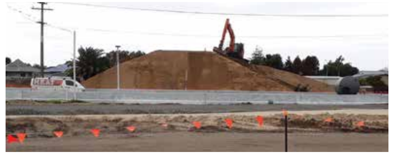
Trial embankment. The trial embankment was constructed in August and during the coming months instrumentation will be monitored to inform how the ground will react to loading, and confirm design predictions for the new embankments. To minimise dust, it has been top soiled and seeded with grass or covered with cloth. Photo by: Brad Wallace, Senior Project Engineer-South
