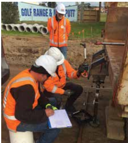
Compaction test. The ground under the road is called subgrade and a strong subgrade contributes to a more durable pavement. In-situ California Bearing Ratio (CBR) testing is used to assess the strength of the subgrade which must meet specific levels before pavement construction can begin. Photo by: Nick Jowsey, Site Engineer
