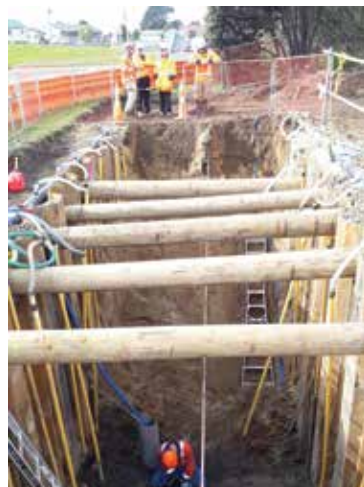
Gas Defect Pit. Installing the new gas lines near SH29A required the pipes to be pulled through an underground tunnel created by a directional drill. Once the pipes were in place they were tested and any damage repaired. The new gas line was commissioned on 30 August. Photo by: Brad Wallace, Senior Project Engineer
