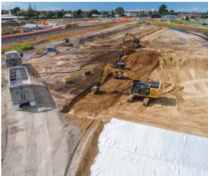
Earth being removed from the vacant land neighbouring SH29A and SH2 near Baypark, to install basal reinforcement, which is a form of ground improvement. Once installed, this is covered with structural fill.
