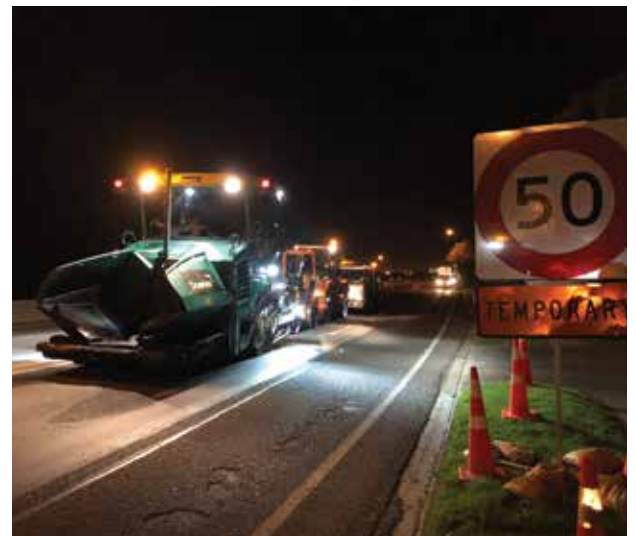
Night works. A paver, roller and truck are lined up ready to begin replacing deteriorated sections of the State Highway 2 road surface during a night shift. Under the right conditions, such as heavy rain events, potholes can form and we ask those travelling through the site to keep to the reduced speed limit for their own safety and the safety of others. Photo by: Evo Lauten, Environmental Coordinator
