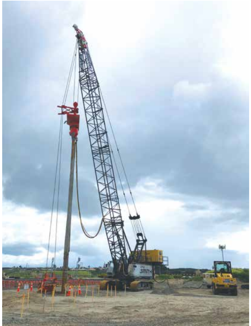
One of the cranes that will construct the 3400 stone columns throughout the site
