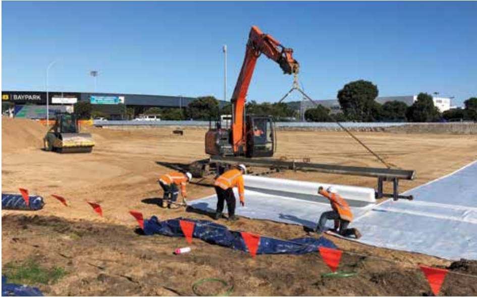
Rolling out grid. Ground improvements are underway on the approach to the new Baypark roundabout, including the installation of geo grid. Photo by: Evo Lauten, Environmental Coordinator
