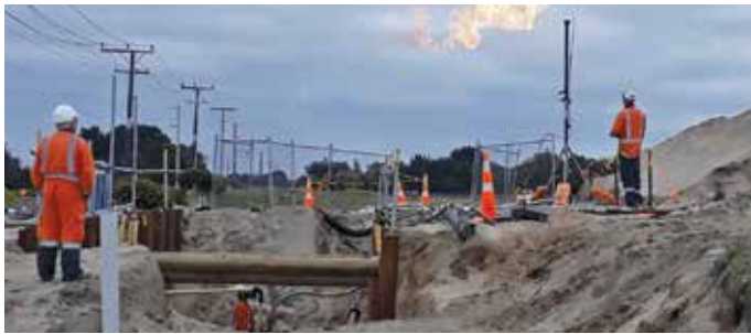
Southern gas pipe relocation. Gas was purged, or burned off, before the new gas line at the southern end of the project was connected into the existing pipe. The new gas line was commissioned at the end of August after completing and testing three new connections. Photo by: Sven Hellqvist, Site Engineer-Structures
