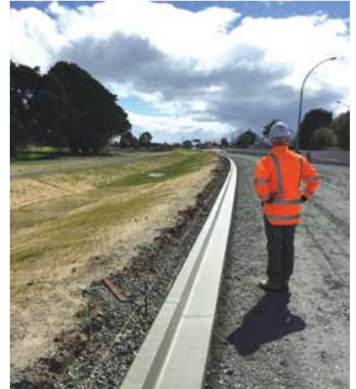
New kerbing. The new city-bound on-ramp starts to take shape with the kerbing installed near the Bayfair intersection. Photo by: Dean Taylor, Construction Manager
