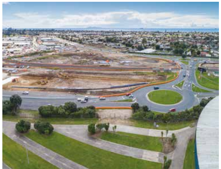
The view over the Baypark and Te Maunga roundabouts shows the extent of the earthworks and ground improvements taking place at this part of the project.
