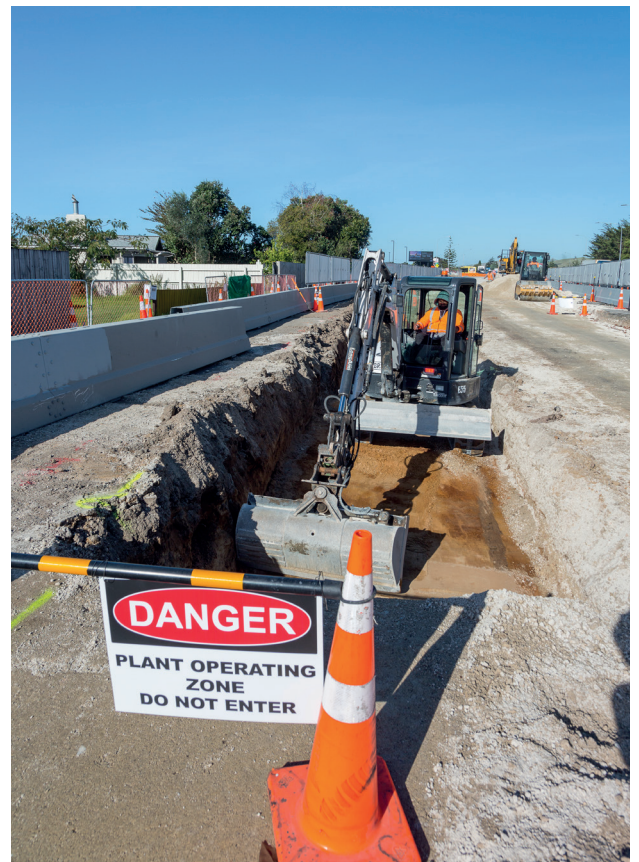
Preliminary ground improvement work is continuing on Maunganui Road between Concord Avenue and Jackson Street with replacement fill being trucked in. Drainage works will start shortly. This work area is compact and close to the traffic lanes, so please take care through this area.
