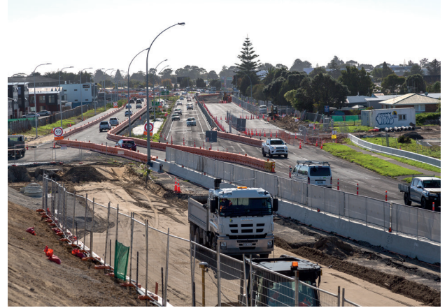
Construction of the new lanes on Maunganui Road between Bayfair and Te Maunga continues.
