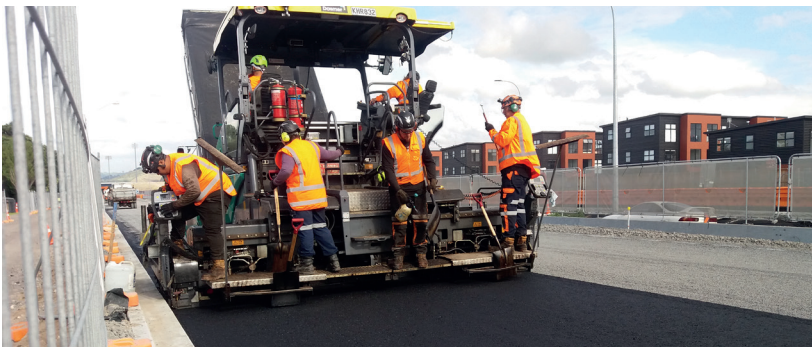
The experienced Downer team on their specialised asphaltting machine lay the first layer of asphalt on Maunganui Road near Exeter Street.
