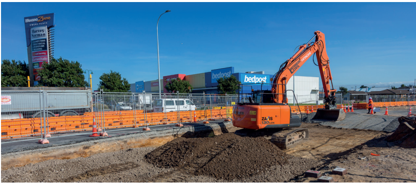
Matapihi Road widening near Golf 360 is continuing. A diversion is in place for pedestrians and cyclists using the underpass. HomeZone and Owens Place are open for business as usual.
