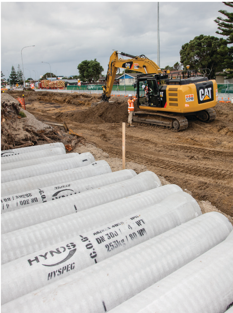
Works continue in preparation for construction of the new north-bound off ramp
