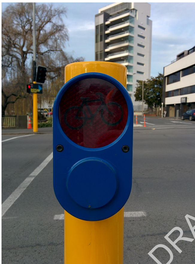
Figure M01 – Cycle call accept indicator (no call present). * Note – Blanking plate fitted to push button as automatic detection installed.
