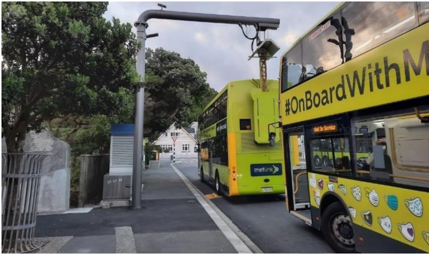
Figure 4: Pantograph electric bus charging facilities, Reef Street, Wellington (Source: Lorelei Schmitt).
