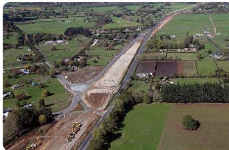
At the northern end of the job: embankments, Pickering Road pond and the roundabout have come a long way in the last few months.
