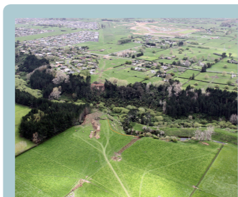
Tree clearing is underway at Karapiro gully and an access track will be formed over the next few months. Select planting post construction of the Viaduct will create a native wetland and provide additional roost locations for bats.
