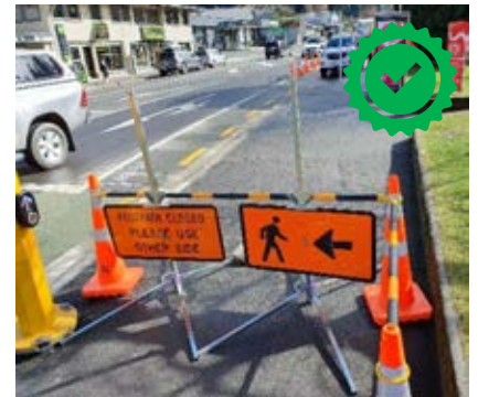
Footpath closure at signalised crossing to allow safe controlled crossing of the road for footpath users. Image Credit xlvi: Danny Wood.
