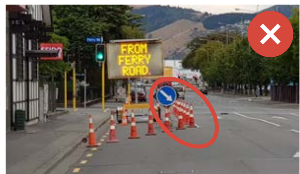
When placing delineation next to traffic lanes – don't put it right up to the lane line/edgeline. Leave space for a small 'shoulder space' for safe cycling (at least 0.5m). Image Credit Ixxix: Glen Koorey.
