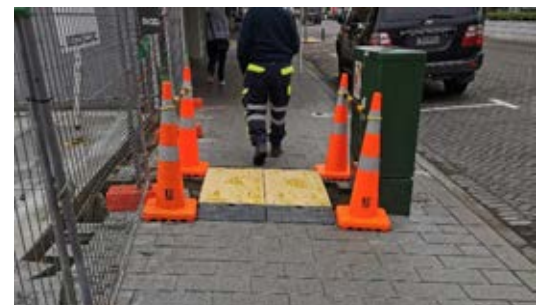
In this instance, high-contrast temporary non-slip covers have been used. These are helpful for people with visual impairments, but there is still a small trip hazard to watch out for. Image Credit Ixiv: Carina Duke.
