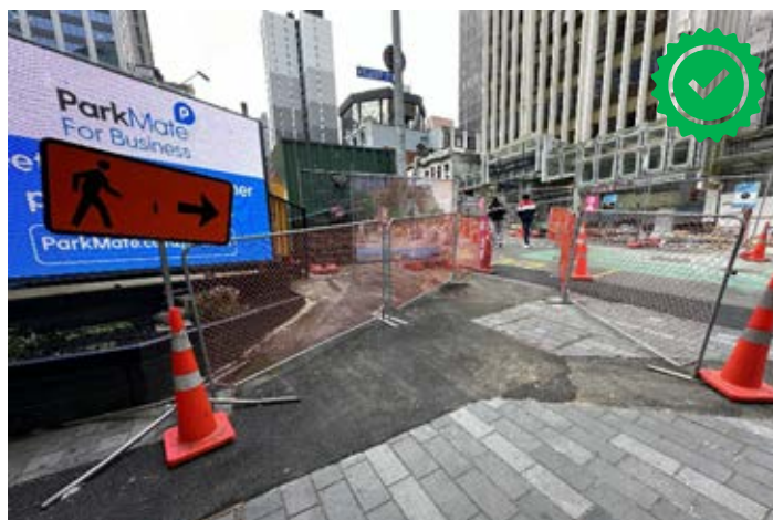
An example of a temporary diverted pedestrian route into a closed road space. One improvement is a few trip hazards that are visible. Image Credit xlv: Parallax.
