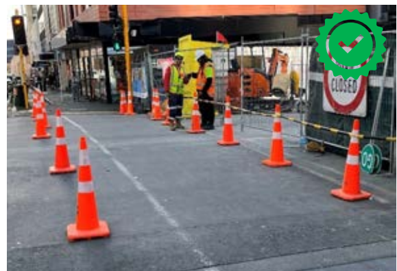
Existing pedestrian crossing maintained with full width and enhanced by some adjacent cones for clarity. Image Credit xli: Betty Mitrova.
