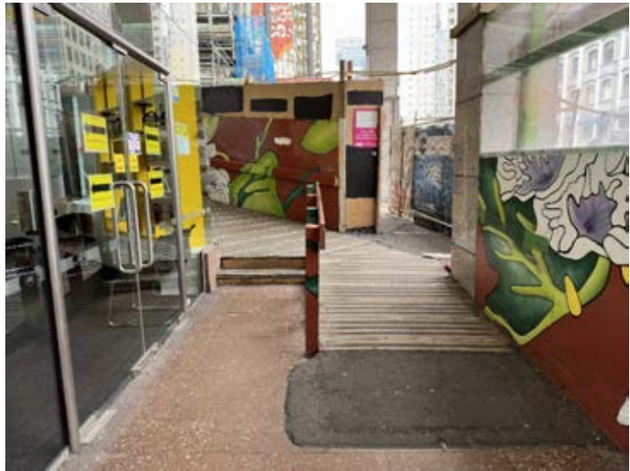
Temporary walkways should always provide accessible routes for those with mobility impairments. In this case, while there are steps – there is a clear and well-formed safe ramp available. Image Credit cvii: Parallaxx.
