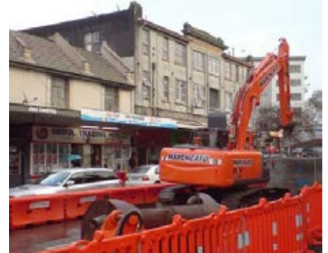
Fencing is particularly important on longer-term worksites, and where heavy machinery is used. Image Credit lxxxvi: Wikimedia Commons.
