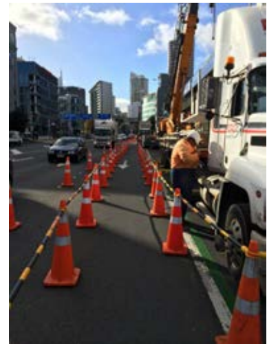
A well-formed temporary walkway is well marked, straight and clear, and separated from other hazards like work activity and live traffic. Image Credit cv: Parallax.
