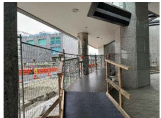
Purpose build bridges can be useful where the geometry and arrangement of pathways is unique and bespoke. Image Credit cxiii: Parallaxx.
