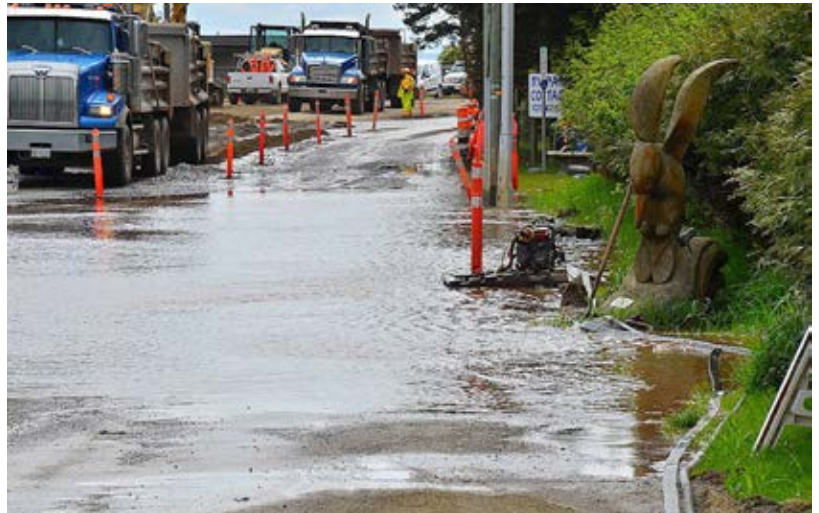
Water can pool in various places, especially in construction environments where the topography has changed. This photo is an extreme version, but even a blocked drain due to construction debris can have an impact on the safety of vulnerable road users in a worksite. Image Credit Ixviii: Campbell River Mirror.
