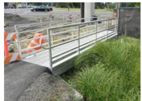
Temporary bridges should be stable and embedded into the pathways either side so there are no trip hazards for users at either end. Image Credit cxiv: Oregon Department of Transport.
