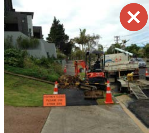
Cone Bars do not stop users and provide little security that access to hazards is prevented. In this instance its clear a user can bypass the control measures into the hazard. Image Credit Ixxvi: Parallax.
