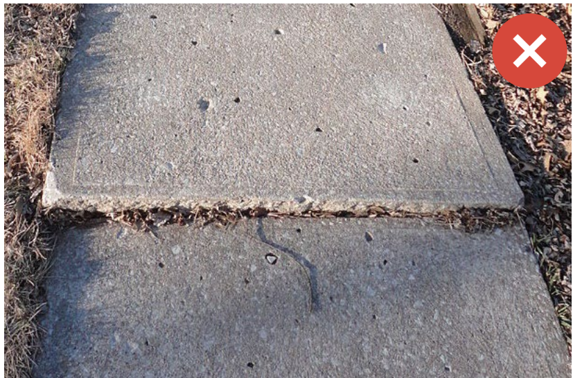
Any footpath (temporary or not) has risk of trips where there are level differences in the surface. Any step thicker than a pencil is a potential trip hazard and should be addressed by fixing the path (preferred), and if not reasonably practicable, delineating and marking the hazard so it is clearly visible. Image Credit cvi: Wikimedia Commons.
