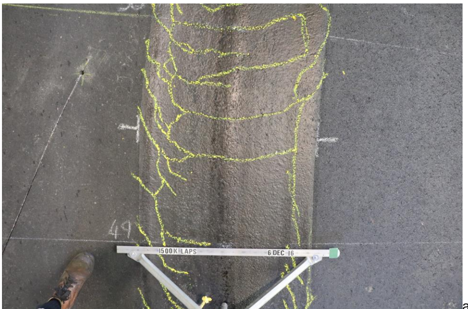
Figure 30 Cracking monitored with Photos
