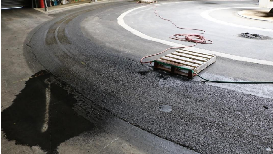
Figure 35 Damp Running conditions
