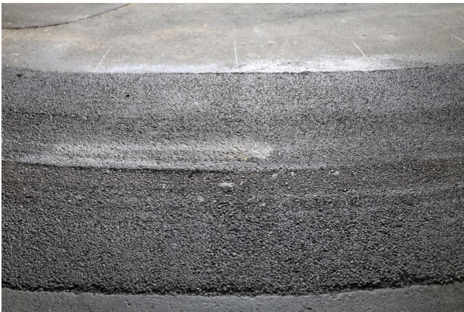
Figure 36 Fines observed pumping to surface in sections A, C and D
