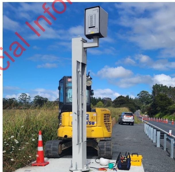
Figure 1: New pole being installed on the Matakana Road average-speed camera corridor near Warkworth
