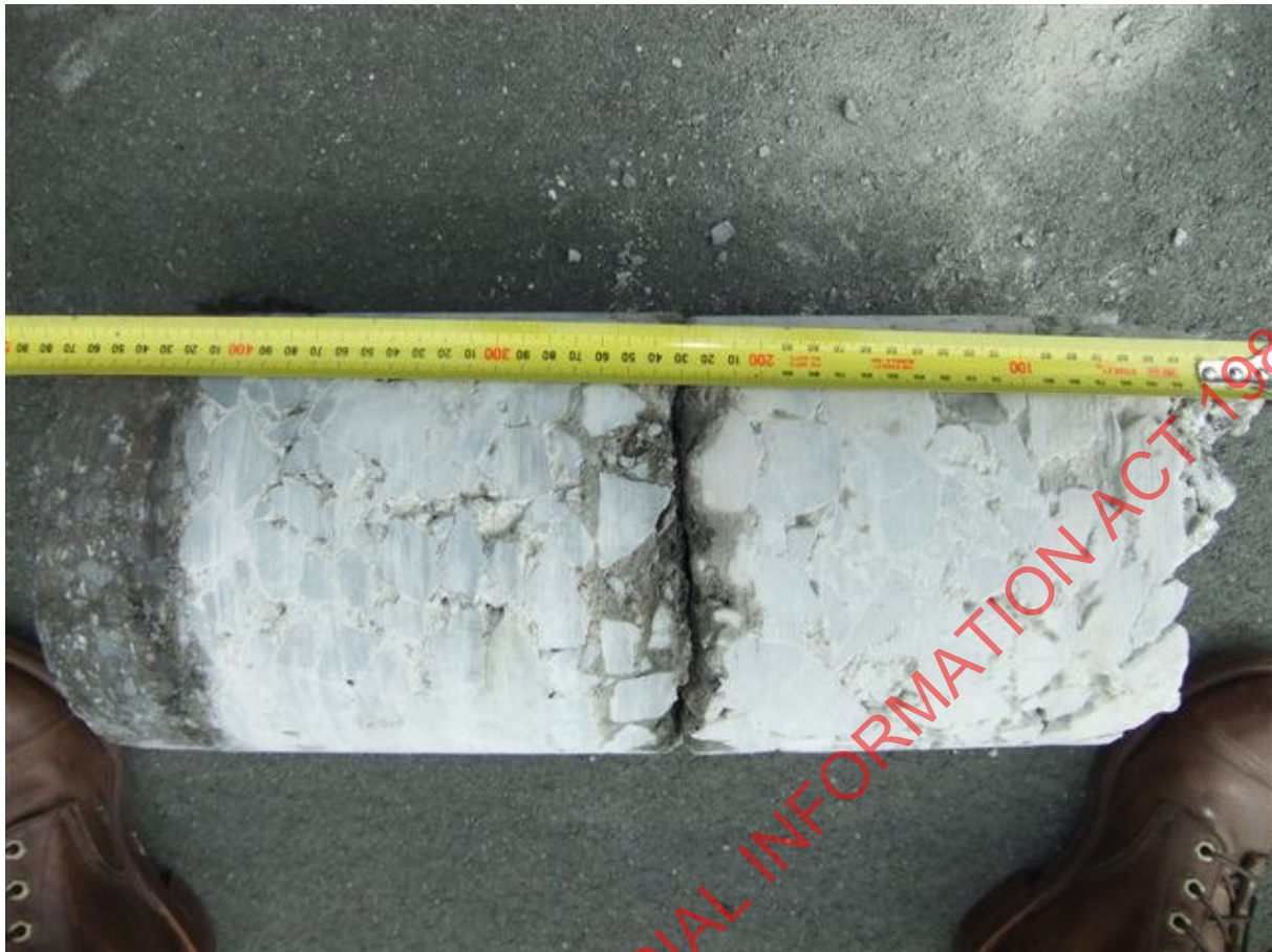
Figure – Photo of debonding between the two stabilised layers.
