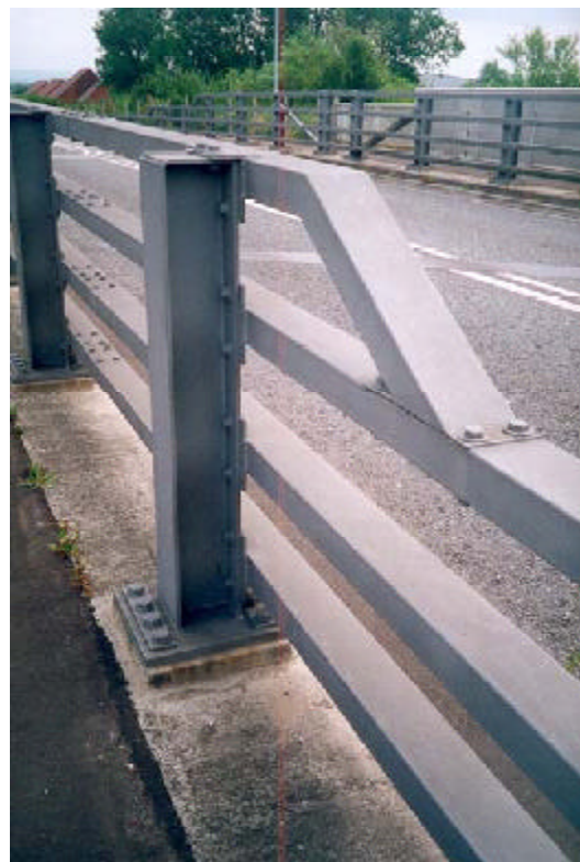
Example of a AS/NZS 3845 crash tested safety barrier (see-through type)
