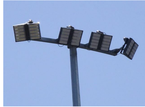
Figure 4-16: Light F with tilt near 45 °s. It produced uplight of 32,100 cd, equivalent to 170 HPS luminaires.
