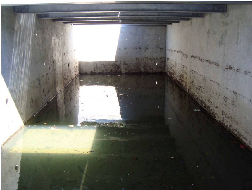
Photo 4: A typical NZTA Sand Filter/Sediment Chamber
