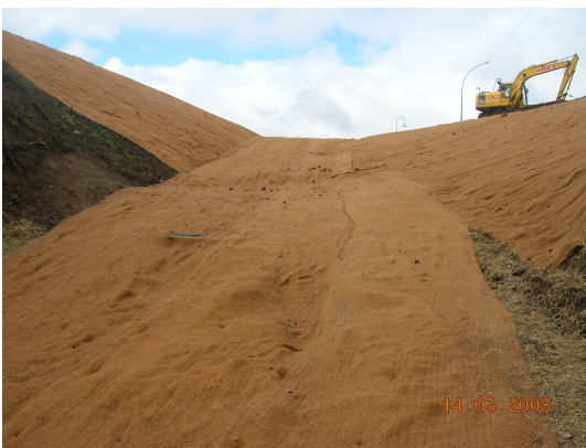
Fibrous geotextile fabric (coconut fibre matting) The geotextile allows to reinstated batter before vegetation is established.
