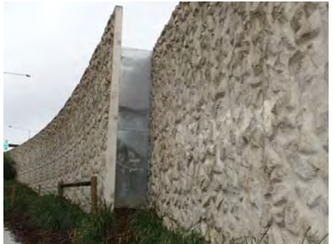
Figure 3.12 Curved noise barrier showing overlaps to delineate change in height and length, Melbourne
