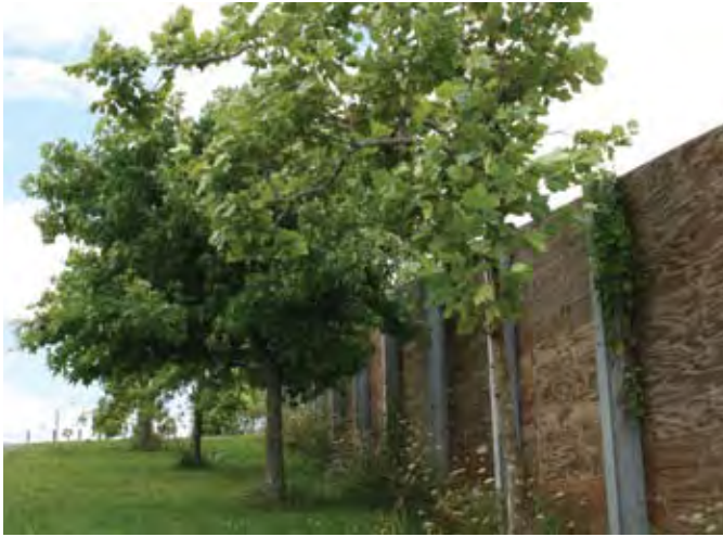
Figure 3.18 The outer face of a noise barrier can be disguised through planting, SH18, Auckland
