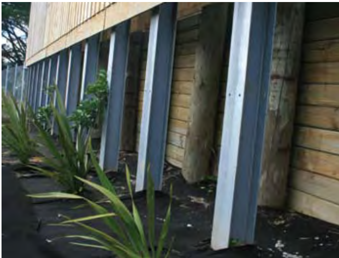
Figure 3.19 Poor detailing of retaining wall, fence and noise wall at Maoro Street, Auckland
