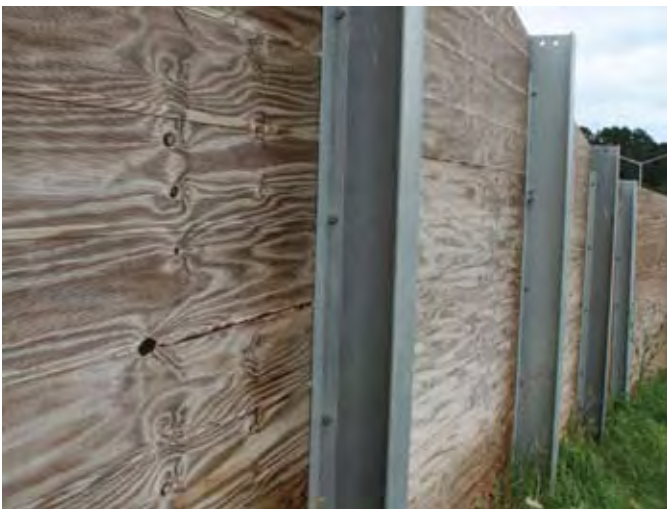
Figure 4.19 Modular marine plywood panels and steel post system have been used on the SH18 Hobsonville motorway extension (non-motorway side view)
