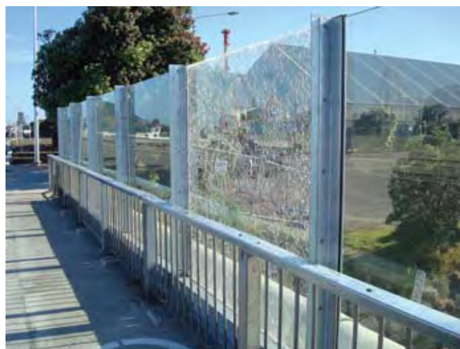
Figure 4.17 Damaged glass noise barrier on Tauranga Harbour Link
