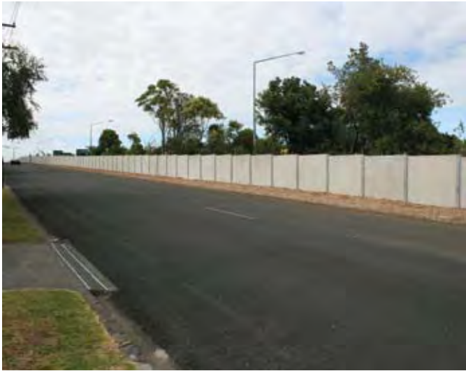
Figure 4.18 Replaceable concrete panels with steel posts have been used on SH1, Market Road, Auckland (pre-landscaping)
