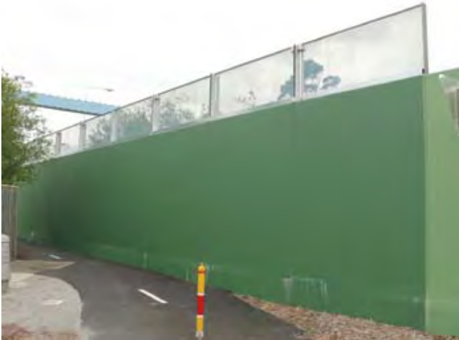
Figure 4.12 Noise barriers can provide dual environmental benefit such as the production of solar power, Tullamarine, Australia
