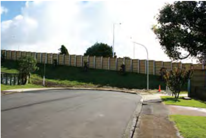
Figure 3.6 Undesirable long shadows can be cast by noise barriers, Maioro Street, Auckland
