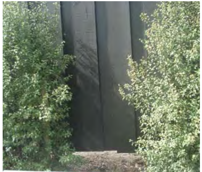
Figure 2.18 Gaps can compromise the overall performance of a noise barrier, Auckland
