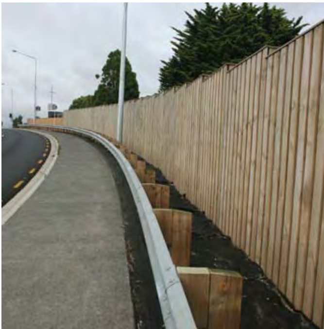
Figure 4.28 Simple timber noise barriers are commonly installed alongside New Zealand roads, Maoro Street, Auckland
