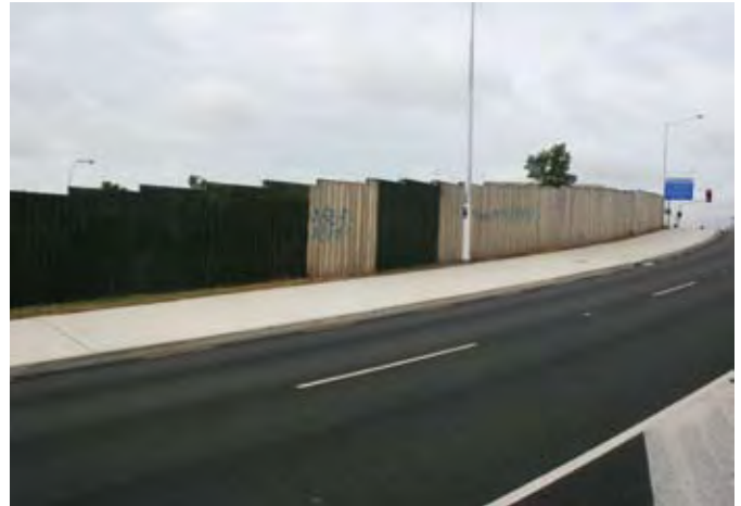
Figure 3.21 Timber barriers should have a paint finish even where graffiti is not a serious risk; leaving some panels unpainted has resulted in a patchwork on this example in Auckland
