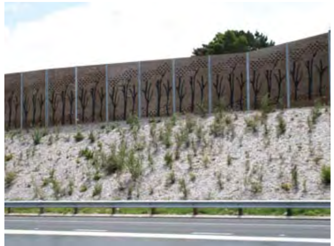
Figure 4.1 Plywood noise barriers on the Hobsonville SH18 extension project have a specified minimum design life of 50 years
