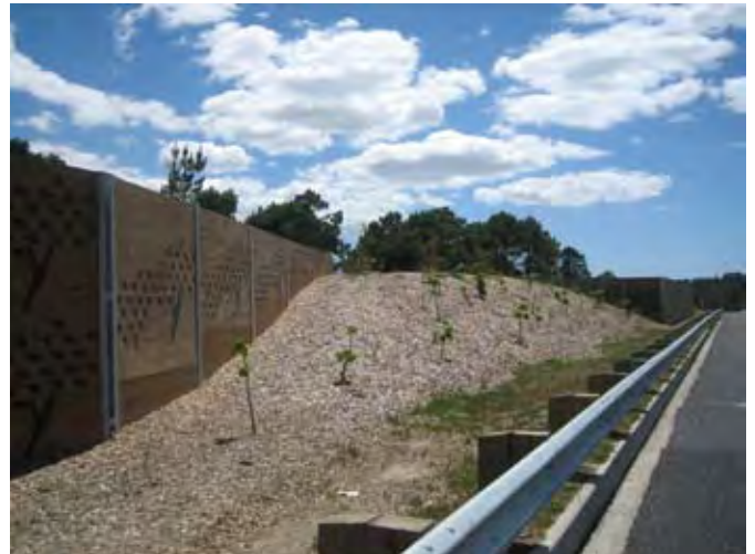
Figure 2.12 SH18 in Auckland Hobsonville has a combination of earth bunds and noise walls to provide an effective noise mitigation solution
