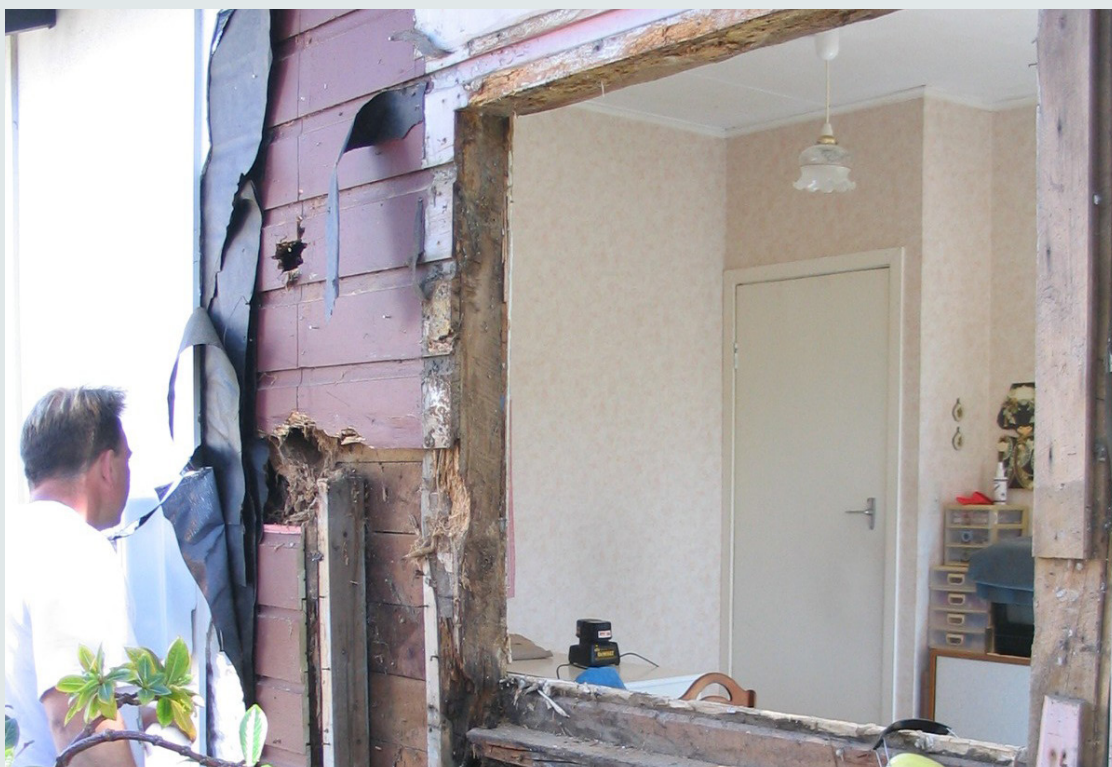
FIGURE 55: EXAMPLE OF ROTTEN FRAMING FOUND WHEN WINDOW REMOVED
