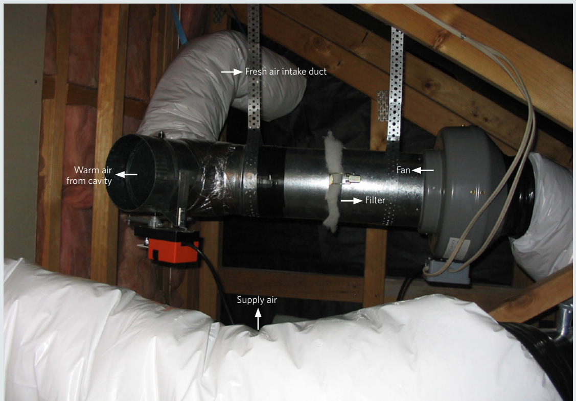
FIGURE 54: FAN AND INSULATED DUCTWORK IN ROOF CAVITY
