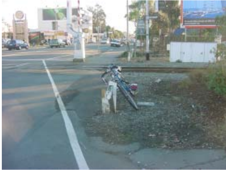
View looking west showing the pedestrian/vehicle conflict area where the footpath terminates and the roadside barrier.
