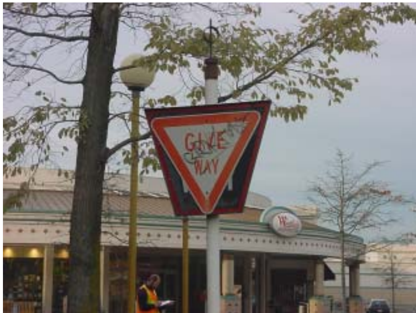
Example of damaged intersection control sign installed over “old” style sign – Kauri Street intersection
