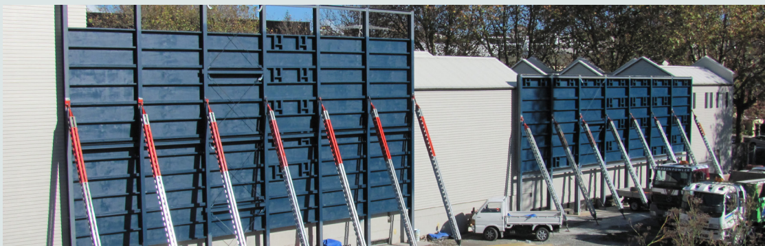
Temporary noise barriers in use at Victoria Park Tunnel
