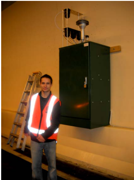
Figure 11: Pillar box housing the particulate monitoring equipment inside the tunnel
