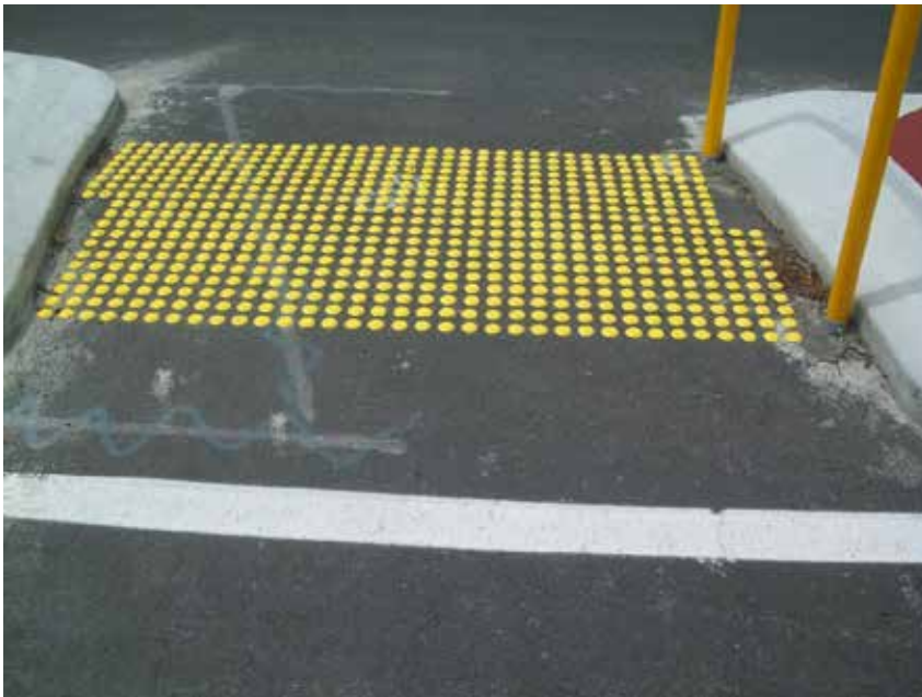
Photo 5.7: Warning indicators correctly installed across the full depth of this pedestrian median island (1.2 - 1.8m deep (Photo: Carina Duke).
