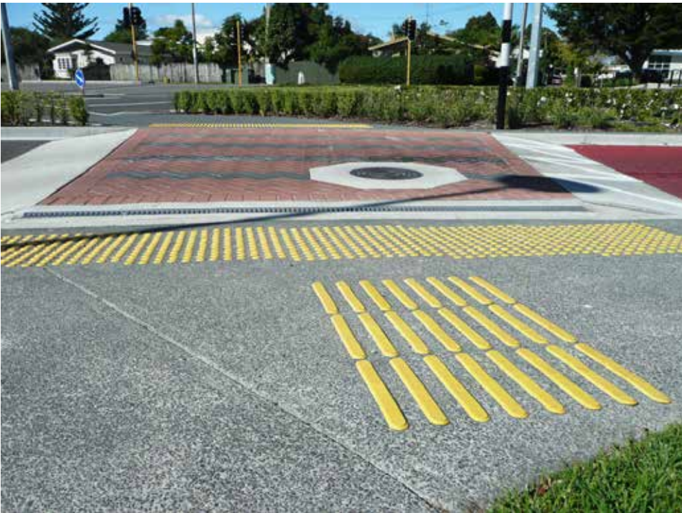
Photo 5.21: This installation shows a textured and raised crossing surface to inform pedestrians who are blind or have low vision of the boundaries of the crossing point. Note the change in texture and colour at the edge of the platform (Photo: Michael Brown).
