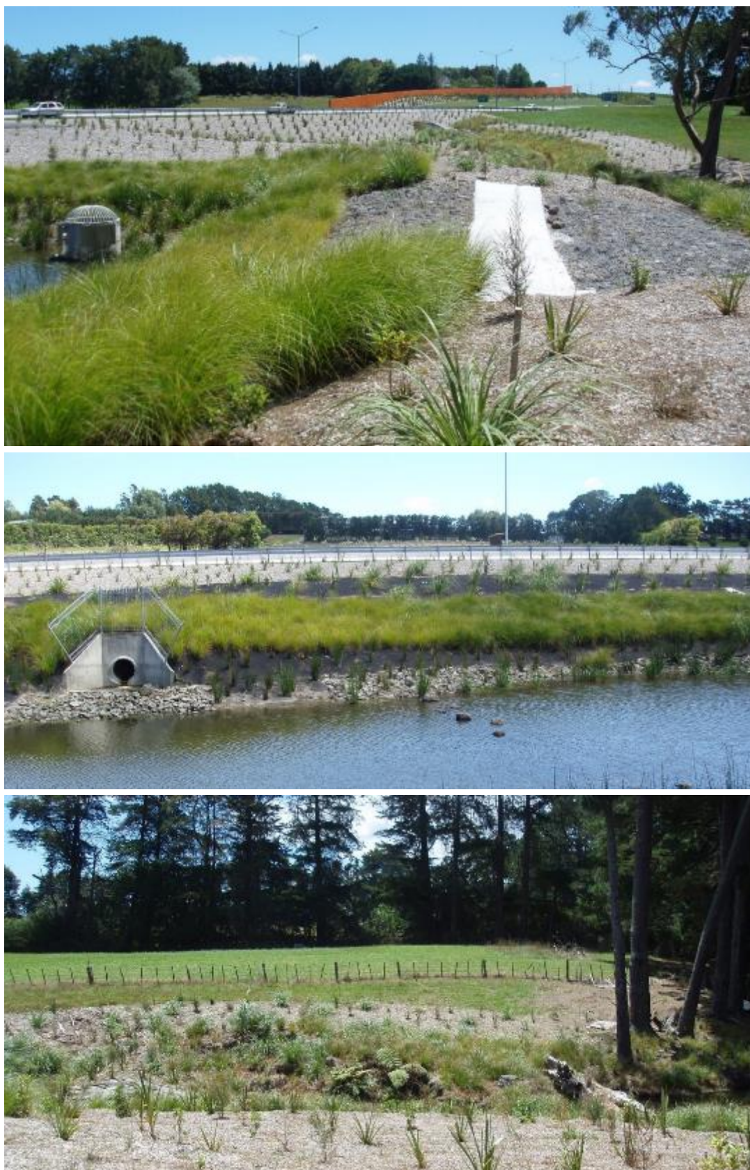
Figure 3.24 Site E. Top: Stormwater pond shortly after construction showing overflows and planting. Middle: Inlet to the stormwater pond. Lower: Pond overflow with nearby retained mature trees and coarse wood habitat features. New plantings are mulched with wood chip. (Photos taken October 2012.)
