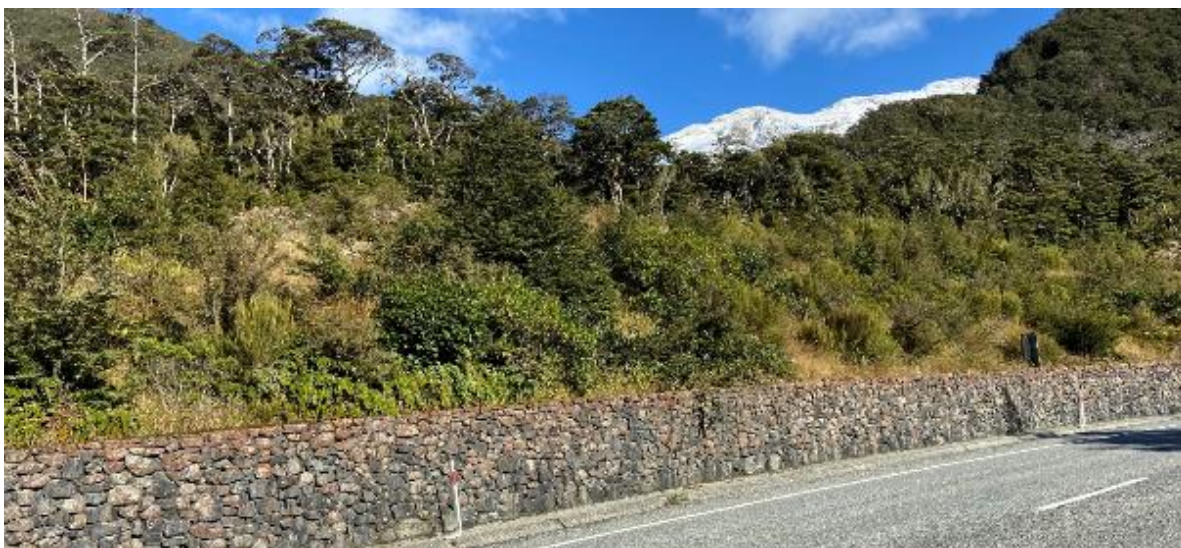
Figure 2.25 This densely vegetated edge in Arthur’s Pass National Park is resistant to weed invasion. The vertical rock walls, which offer no sites for seedling germination, and the concrete kerb with no gravel margin have eliminated areas vulnerable to weed invasion. (Photo taken April 2021.)
