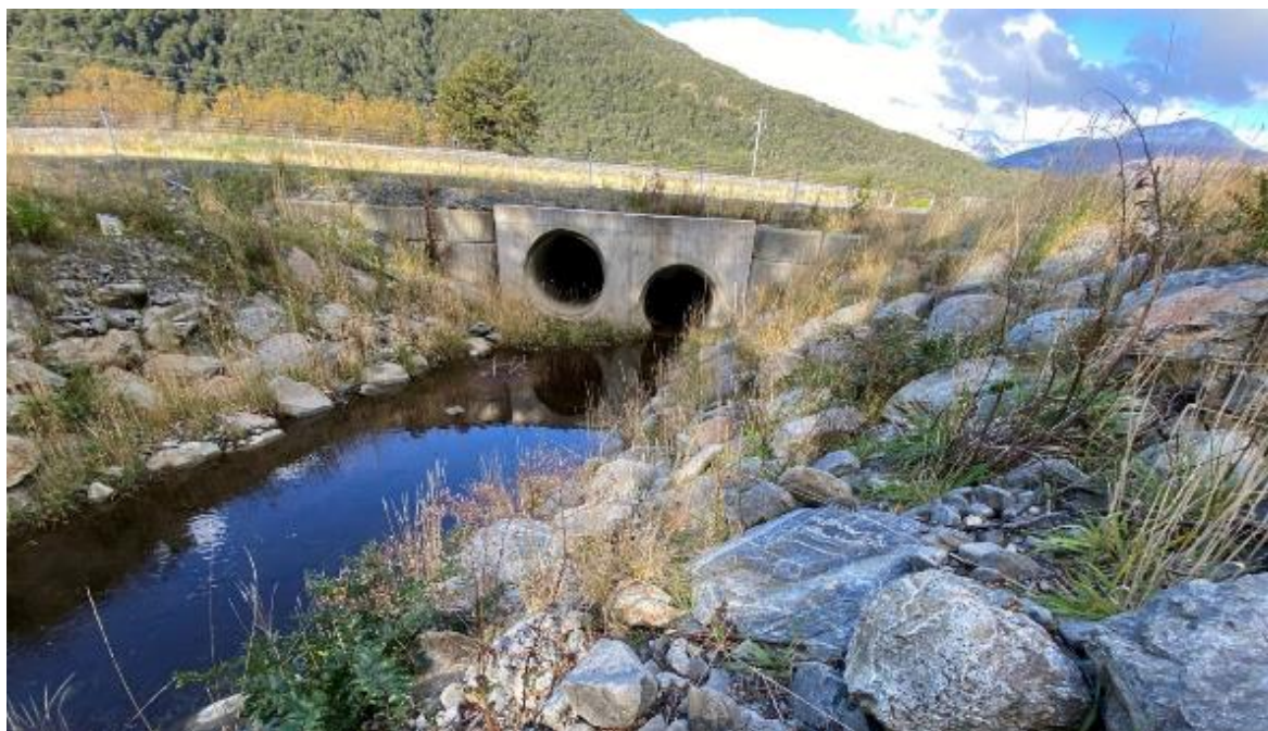
Figure 4.20 New culverts on the Mingha Bluff section of SH73 near Arthur's Pass are designed to cater for intense alpine rainfalls (upper pipe and boulder lining) and year-round fish passage (lower pipe). The new channel is partly shaded by adjacent forest, but has low riparian vegetation cover 3 years after opening, although tutu is establishing (left foreground). (Photo taken April 2021.)
