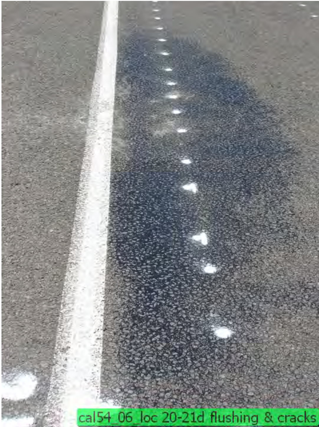
Figure A.1 Photograph 1, CAL- 54, 19 January 2007, loc 20- 21d flushing and cracking
