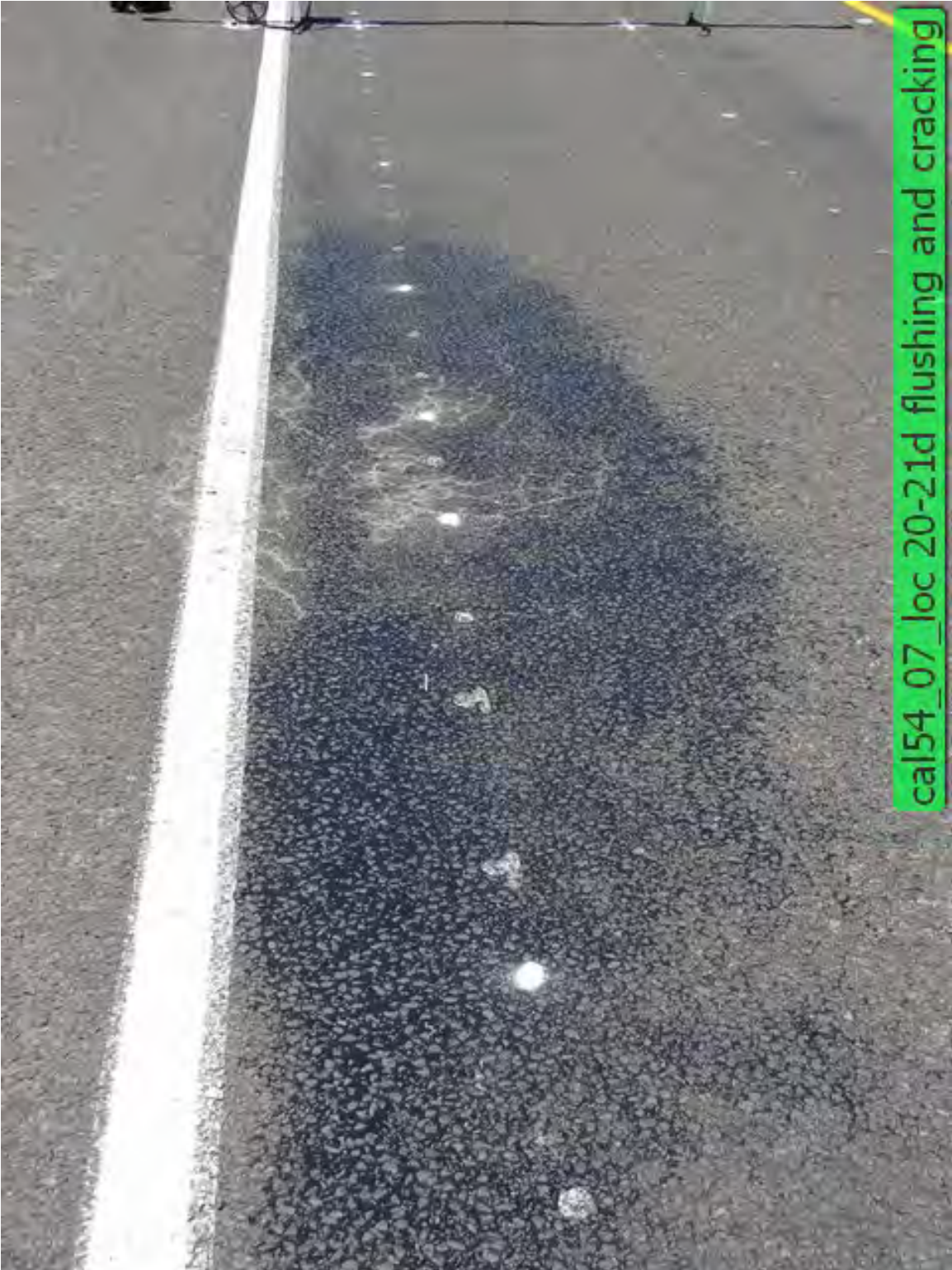
Figure A.2 Photograph 2, CAL- 54, 22 November 2007 loc 20- 21d flushing and cracking
