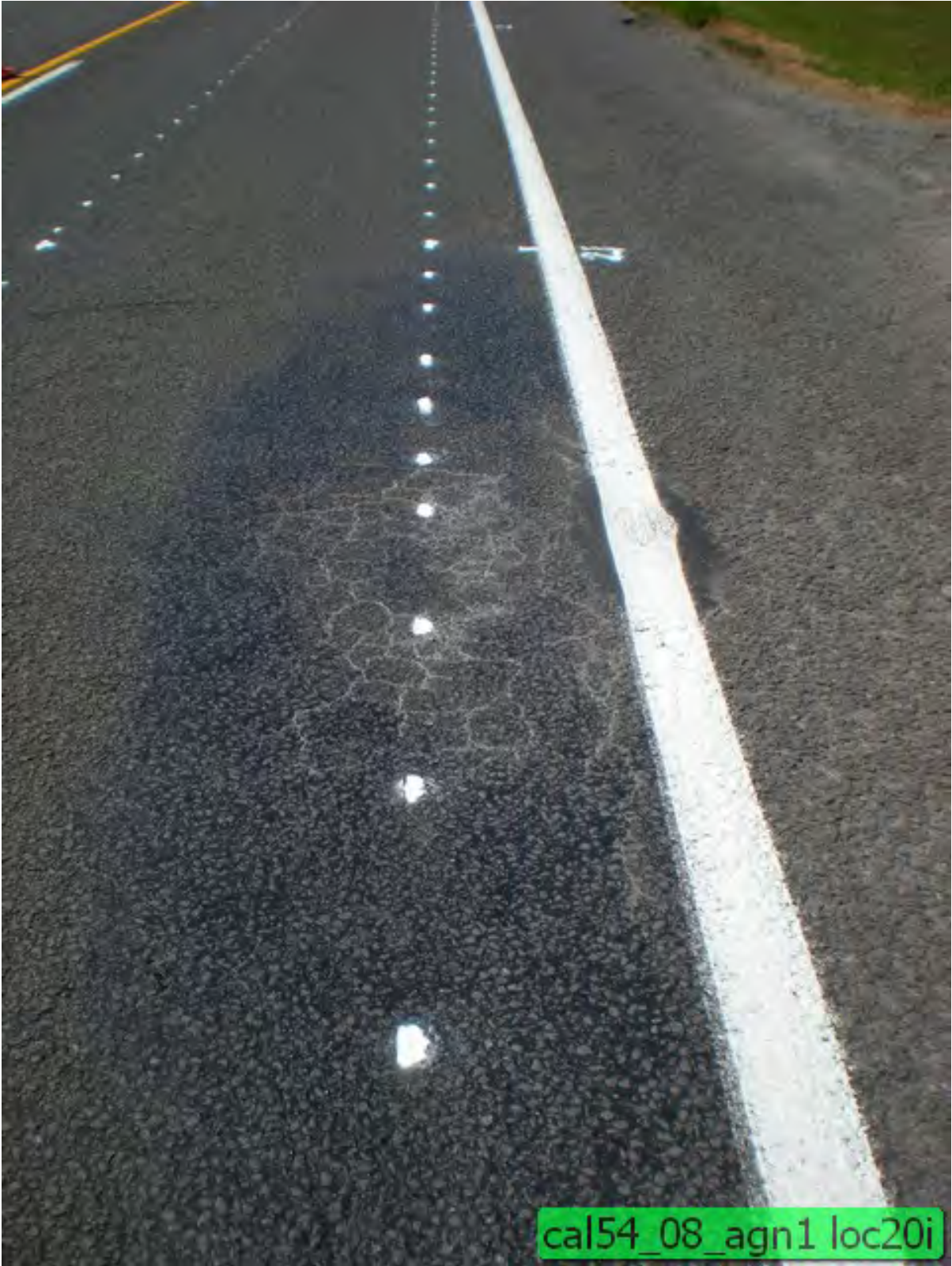
Figure A.3 Photograph 3, CAL- 54, 21 November 2008 loc 20- 21d flushing and cracking
