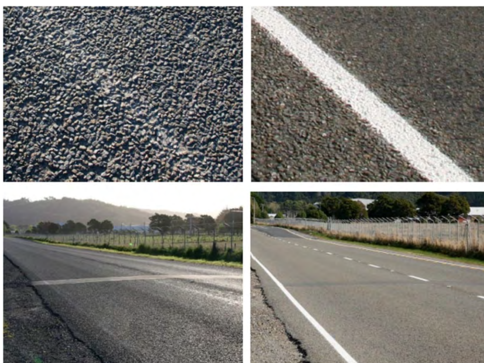
Figure 3.1 Example roadmarkings before (left 38 mcd/m 2 /lux) and after (right, 142 mcd/m 2 /lux) an upgrade
