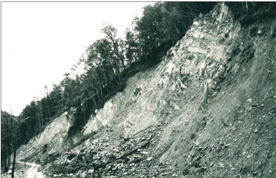
Figure A.14 One of the many steep unsupported SH6 road cuts in the upper Buller Gorge which were badly damaged by rock and debris falls during the Inangahua earthquake. In this photo much of the rock fall debris has been cleared away, allowing the highway to be re-opened to one-lane traffic 10 weeks after the earthquake.
