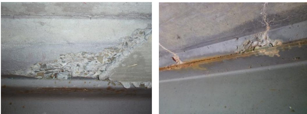
Figure 3.11 Examples of distress signs noted
