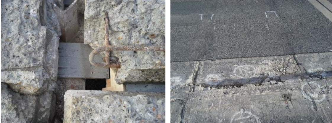
Figure 3.12 Breakage of the grout around the welded angle
