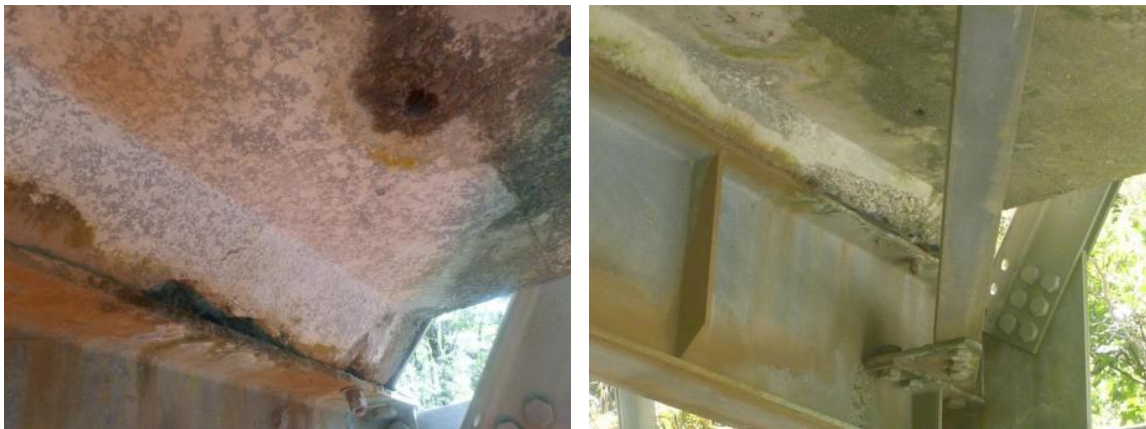
Figure 3.13 Example of failed bolts providing the shear connection between the concrete slab and steel girder
