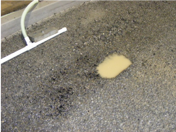
Figure 3.2 Test 2 – first failure
