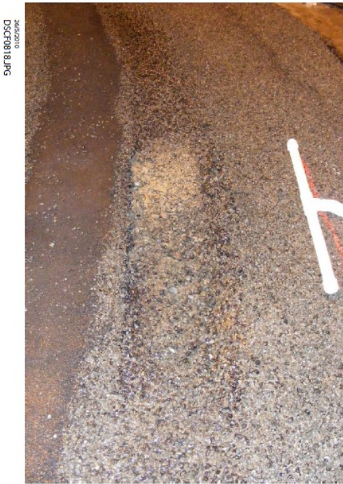
Figure 2.18 Test 1 – first failure
