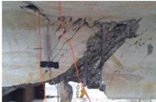
(b) Crack pattern during loading
