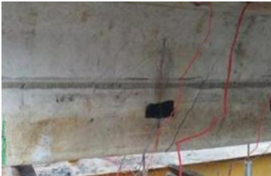
(a) Crack pattern during loading
