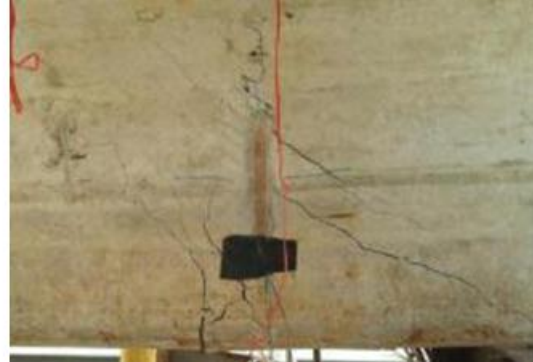
(b) Crack pattern at failure
