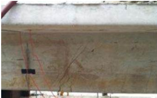
(a) Crack pattern during loading
