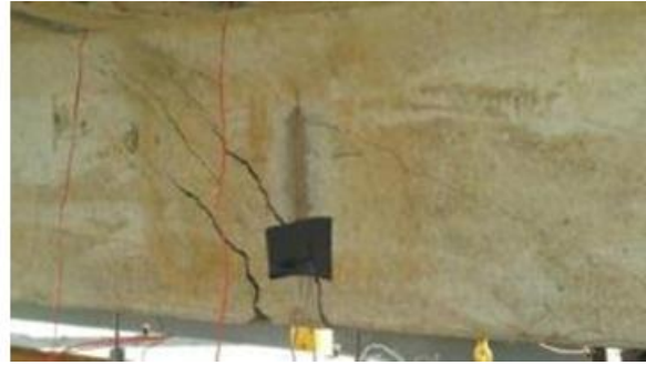
(b) Dominant crack at failure
