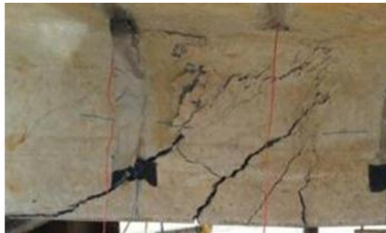
(b) Dominant crack at failure
