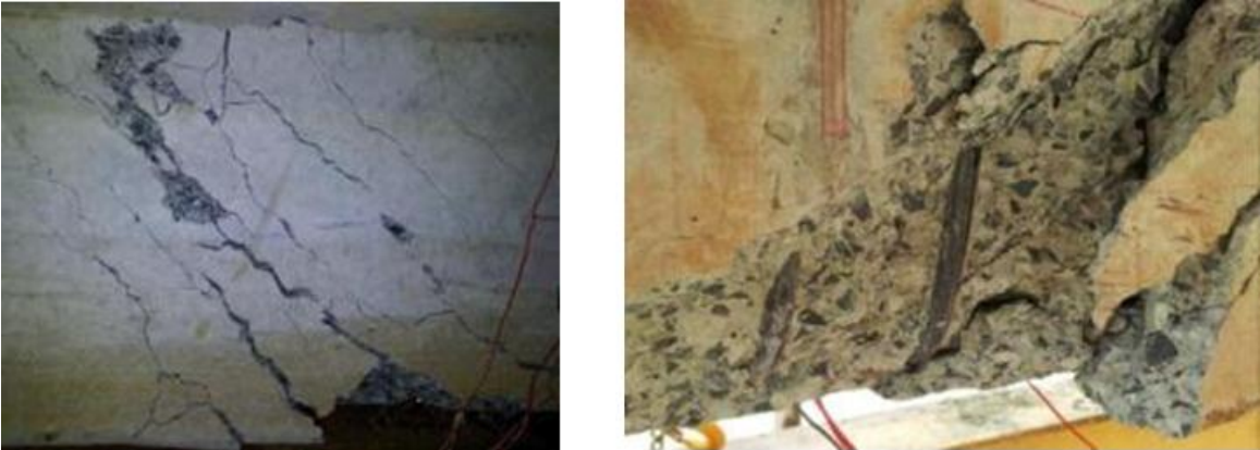
(c) Dominant crack at failure, opposite side of web (d) Web damage at failure
