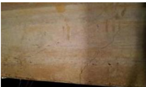
(a) Cracking during loading
