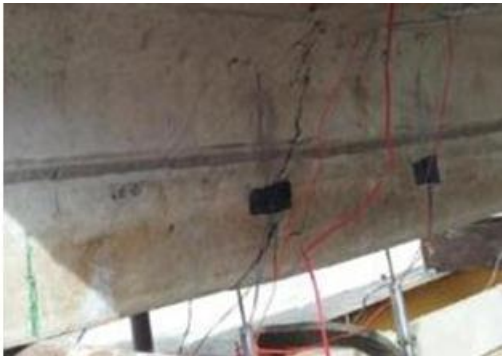
(b) Dominant crack at failure
