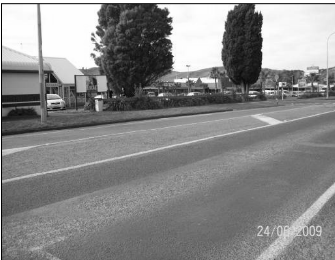
Figure 4.21 View of site B10, showing an area of flushing
