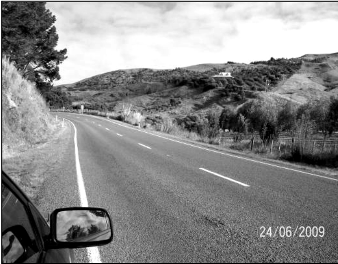
Figure 4.20 View of site B9, showing scabbing
