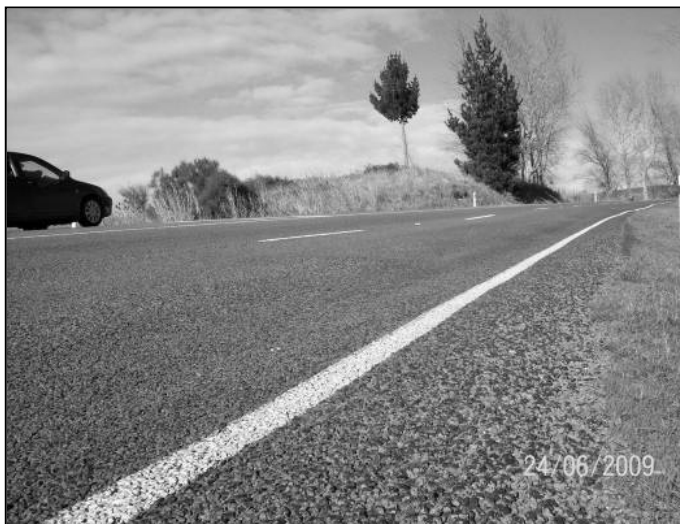
Figure 4.7 View of site B3, showing rutting
