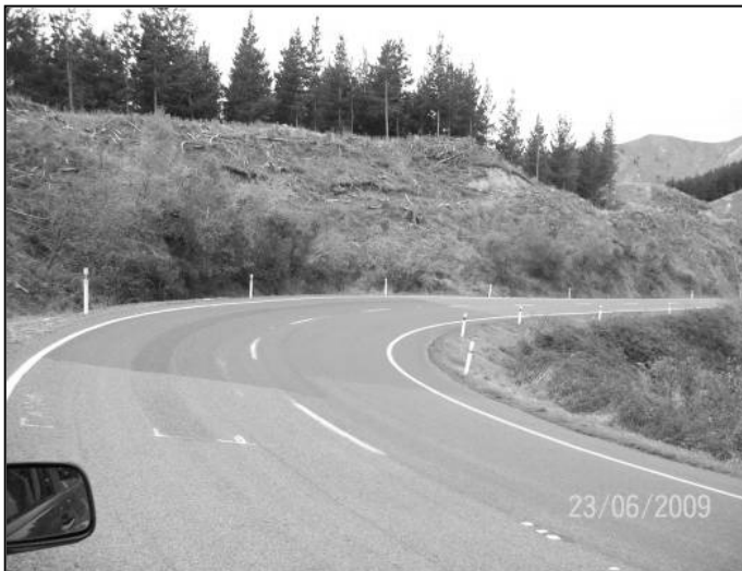
Figure 4.41 View of site C11, showing patchwork repairs and wide flushing on a curve
