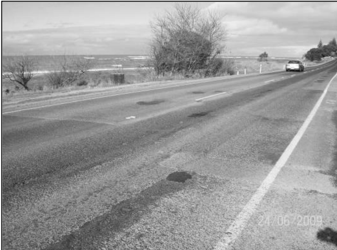
Figure 4.18 View of site B8, showing a range of problems contributing to pavement roughness
