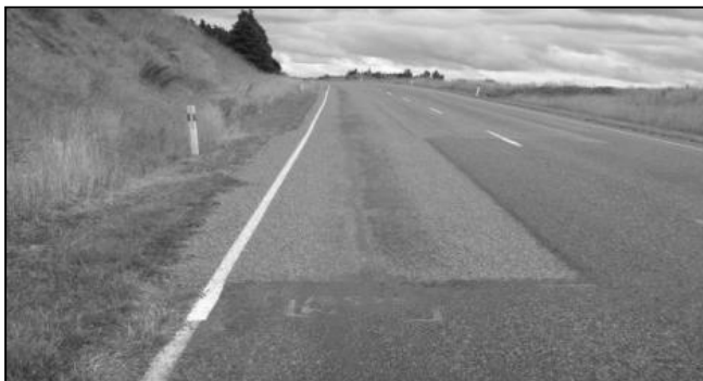
Figure 4.53 View of site D1, showing another area of patchwork repairs
