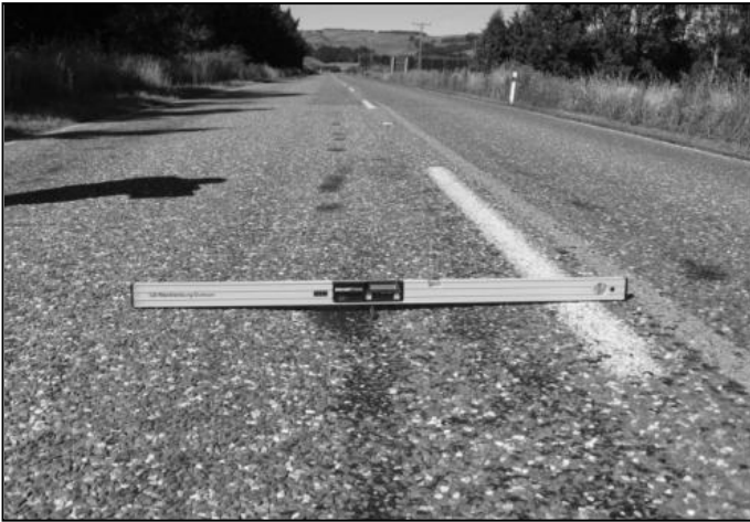
Figure 4.67 View of site D8, showing the depth of the rutting
