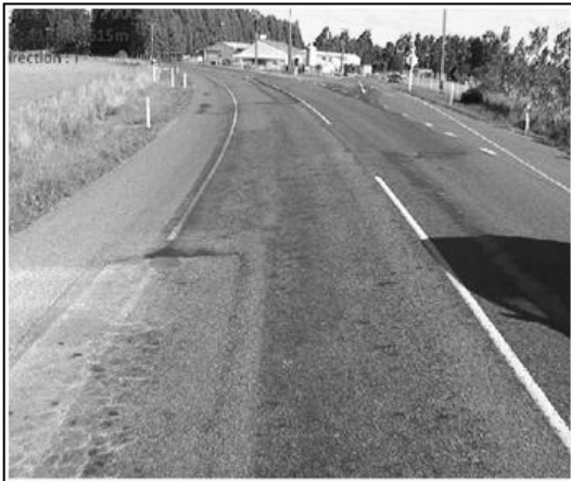
Figure 5.41 Another section of the inspection length in site D2 (RP 1145/6615), showing patchwork repairs, flushing and other evidence of poor pavement condition
