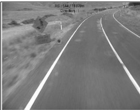
Figure 5.35 Typical section of site C10 (RP 544/11,378 increasing), showing flushing
