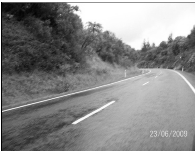
Figure 4.50 View of site C18, showing the extensive flushing evident at this site
