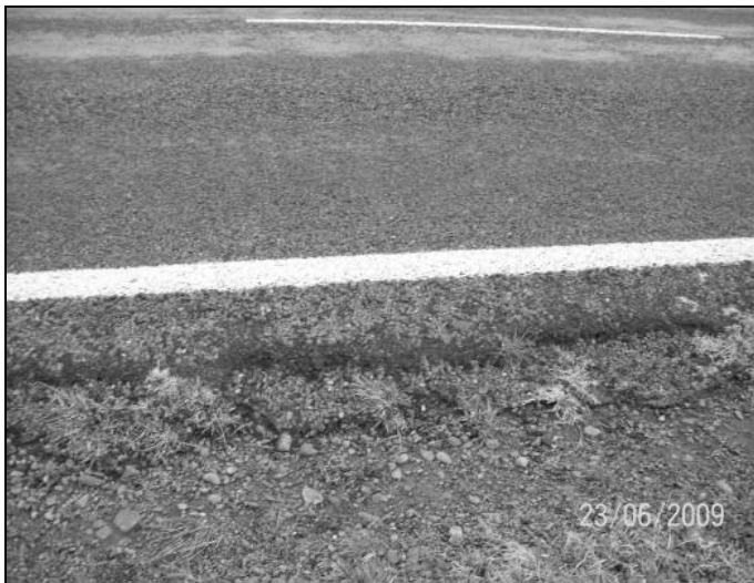
Figure 4.42 View of site C13, showing shape loss at the edge of the seal
