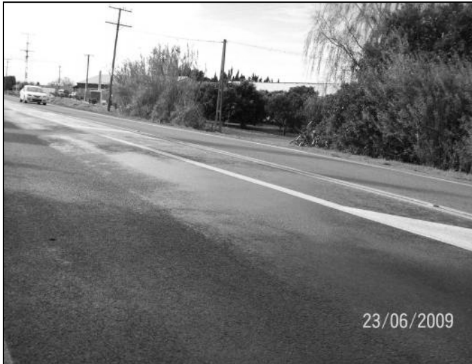
Figure 4.35 View of site C7, showing shape loss and flushing
