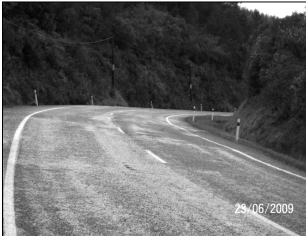
Figure 4.51 View of site C18, showing shape loss and patchwork repairs
