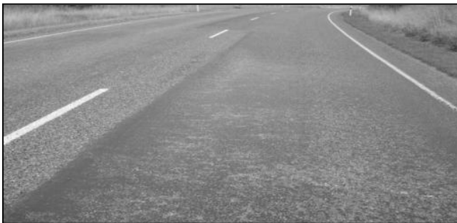
Figure 4.52 View of site D1, showing patchwork repairs and flushing
