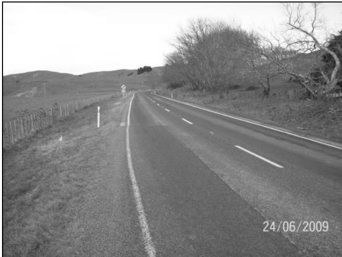
Figure 4.12 Alternate view of site B5, showing flushing and patchwork repairs
