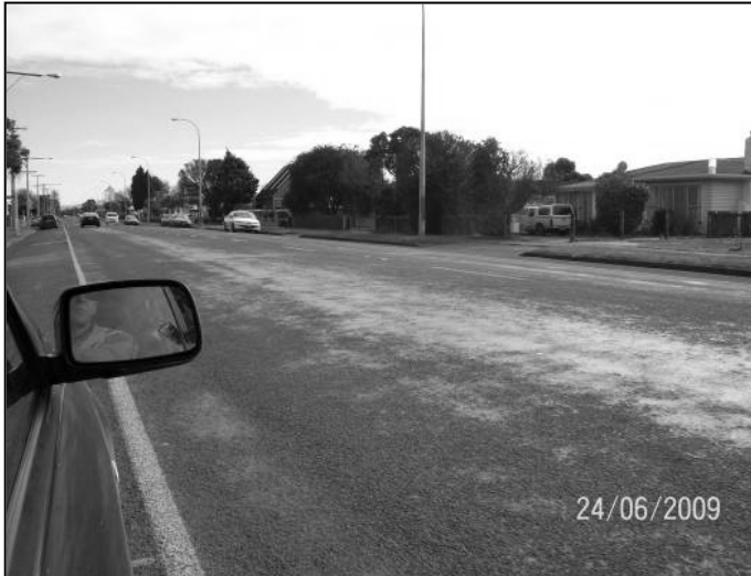
Figure 4.22 View of site B10, showing flushing
