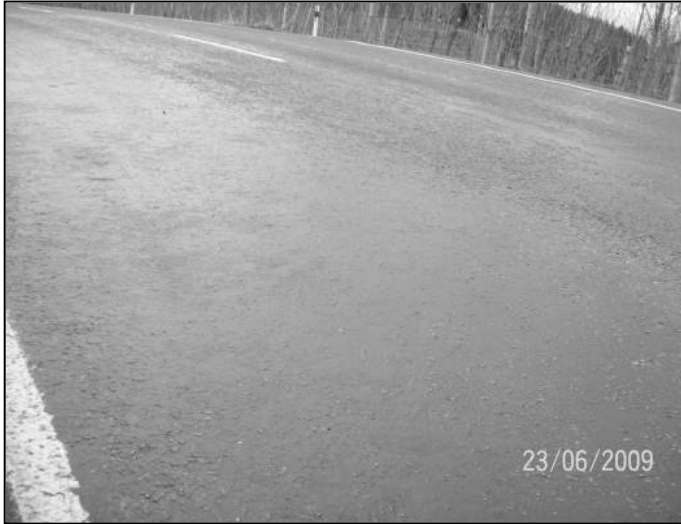
Figure 4.40 View of site C11, showing flushing on the full width of the road
