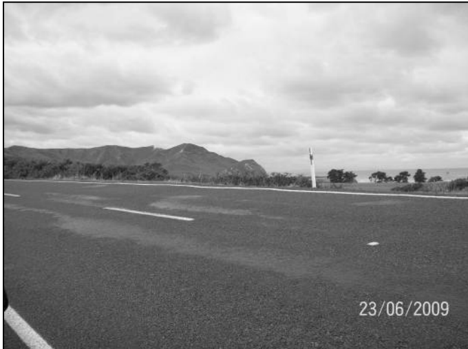
Figure 4.38 View of site C10, showing several areas of flushing
