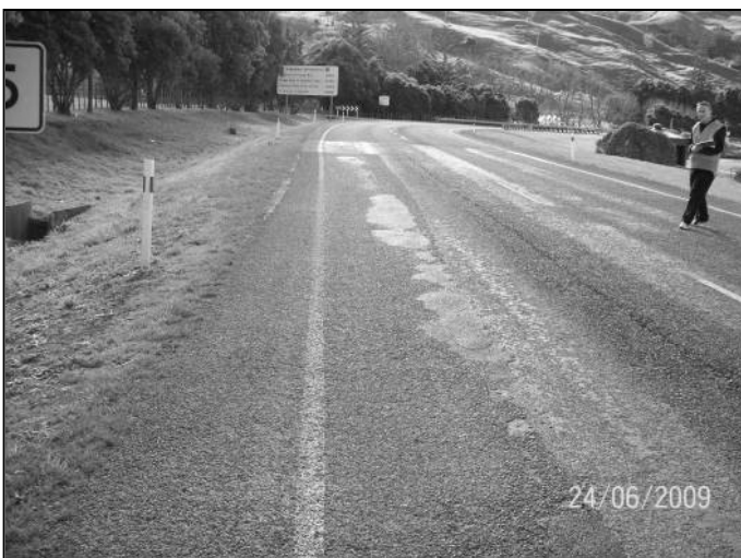
Figure 4.17 View of site B8, showing flushing and patchwork repairs
