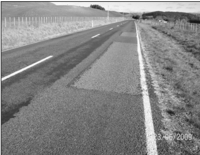
Figure 4.23 View of site C1, showing patchwork repairs and flushing
