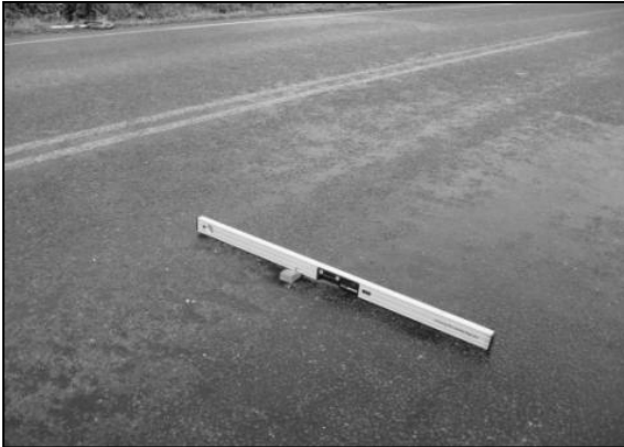
Figure 4.71 View of site D10, showing the depth of the rutting
