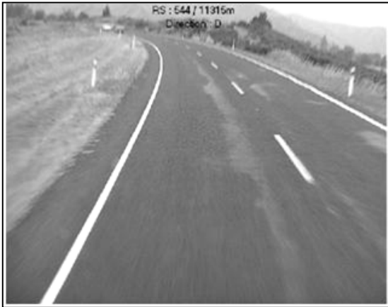
Figure 5.36 Typical section of site C10 (RP 544/11,315 decreasing), again showing some areas of flushing
