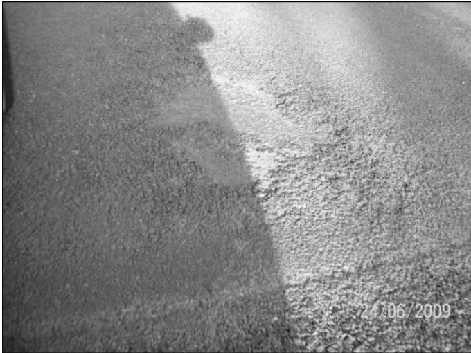
Figure 4.6 View of site B2, showing a close-up view of scabbing/chip loss
