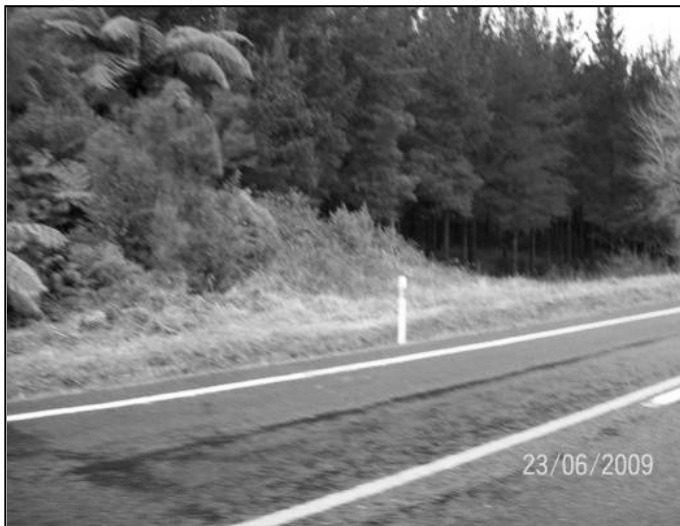
Figure 4.46 View of site C16, showing flushing
