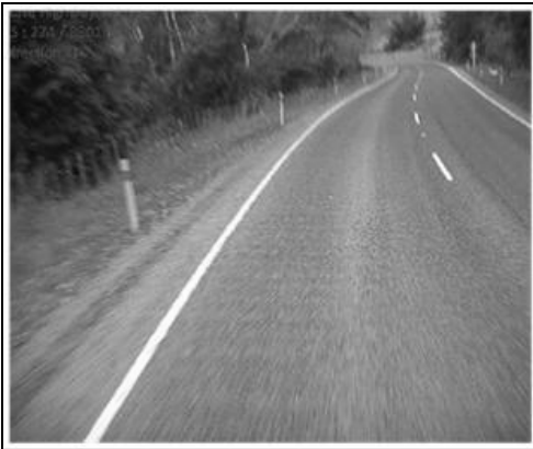
Figure 5.11 Typical distress in site B2 (RP 8801), showing evidence of corrugation
