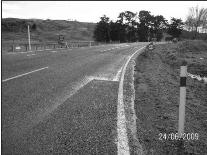
Figure 4.10 View of site B4, showing an example of patchwork repairs
