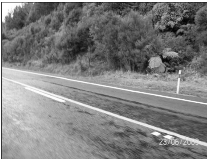
Figure 4.47 View of site C16, showing patchwork repairs and flushing
