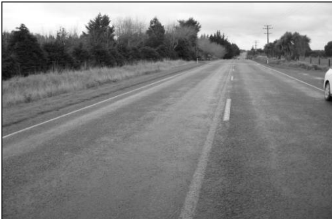
Figure 4.70 View of site D10, showing extensive flushing in the wheeltracks
