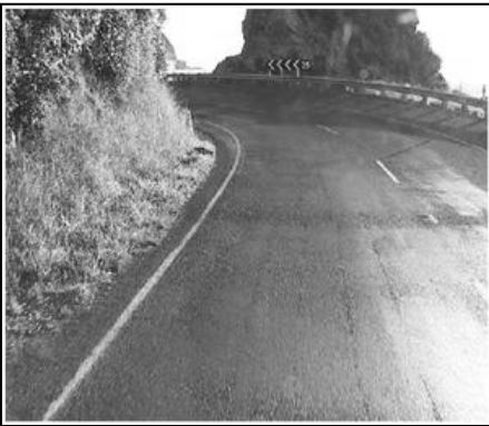
Figure 6.52 Another view of the inspection length in site E1 (RP 15,531 decreasing), showing flushing
