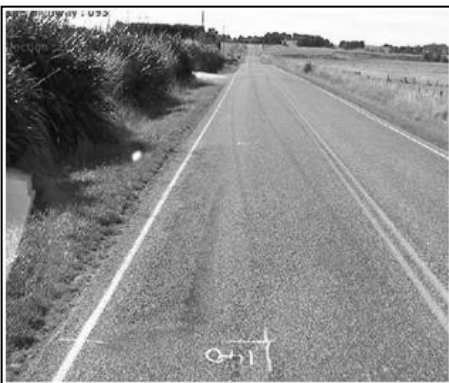
Figure 5.44 Typical section of site D6 (second half, shown in figure 5.43): RP 8675 decreasing
