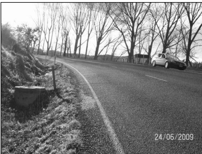
Figure 4.5 View of site B2, showing chip loss at the edge of the pavement
