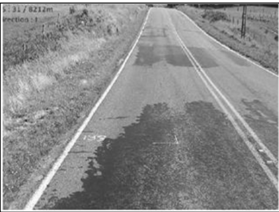
Figure 5.47 Another typical section of the first half of site D6: RP 8210 increasing, showing generally poor pavement surface condition
