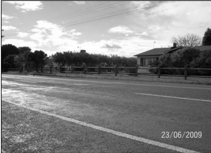
Figure 4.33 View of site C6, showing more flushing
