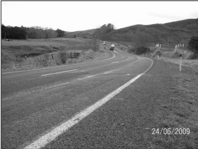
Figure 4.16 View of site B7, showing extensive rutting
