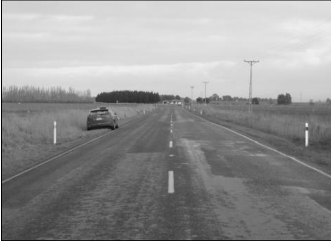
Figure 4.69 View of site D9, showing the overall poor condition of the pavement
