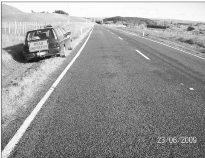
Figure 4.24 View of site C1, showing minor flushing
