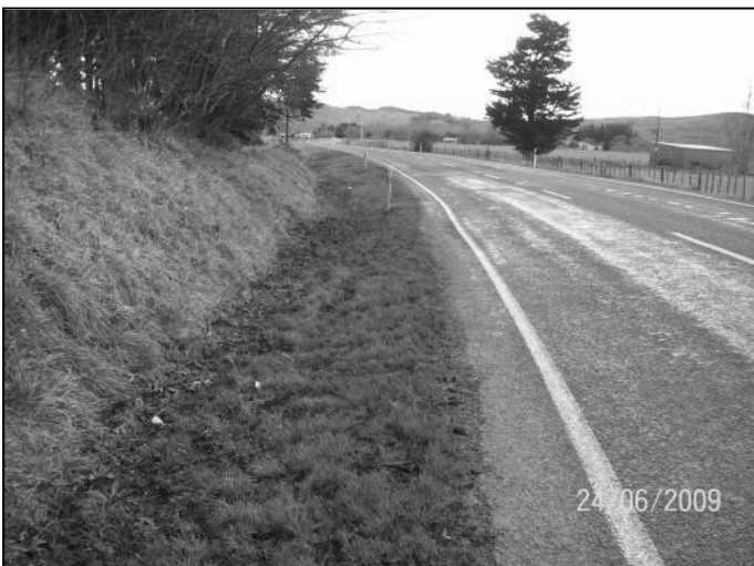
Figure 4.11 View of site B5, showing flushing and shape loss
