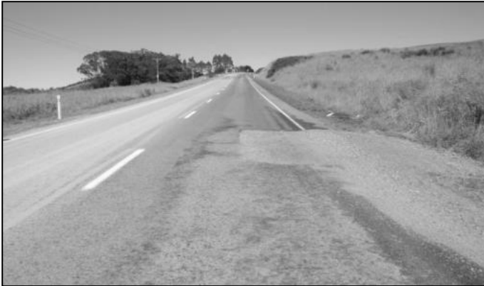
Figure 4.59 View of site D4, showing the overall poor condition of the pavement surface
