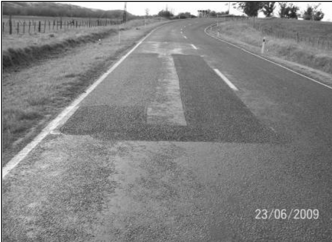
Figure 4.31 View of site C5, showing patchwork repairs and flushing
