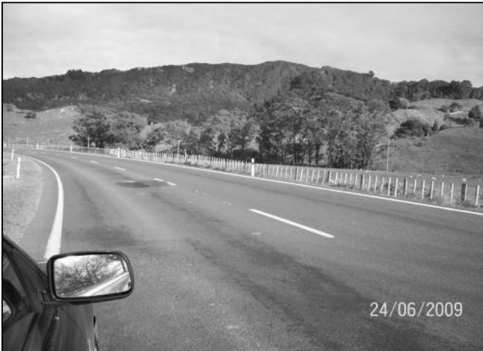
Figure 4.4 View of site B1, showing an extended area of flushing
