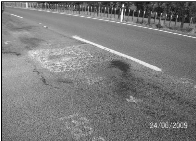
Figure 4.3 View of site B1, showing patchwork repairs and flushing
