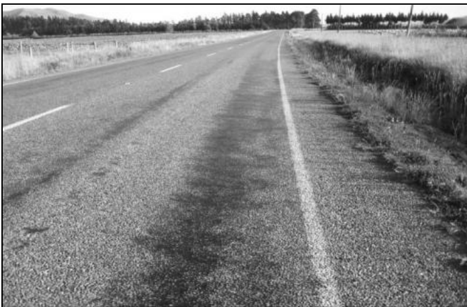
Figure 4.64 View of site D7, showing flushing in the wheelpaths
