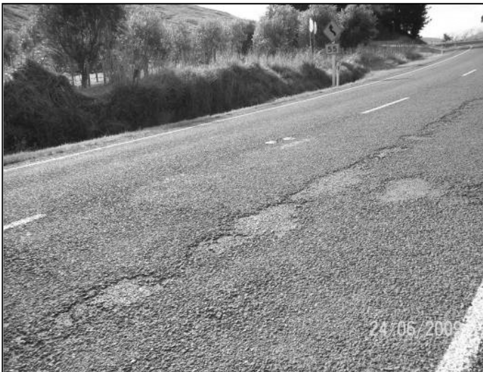
Figure 4.19 View of site B9, showing scabbing
