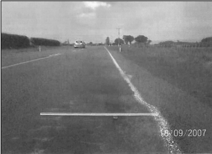
Figure 4.1 View of site 2, showing evidence of flushing and other areas of poor condition
