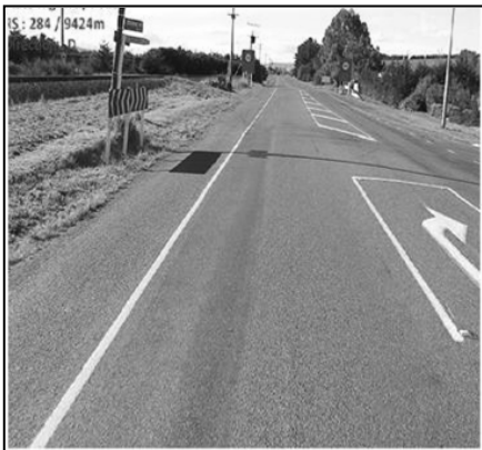
Figure 5.70 Alternative view of inspection length 2 in site E2: RP 284/9422 decreasing
