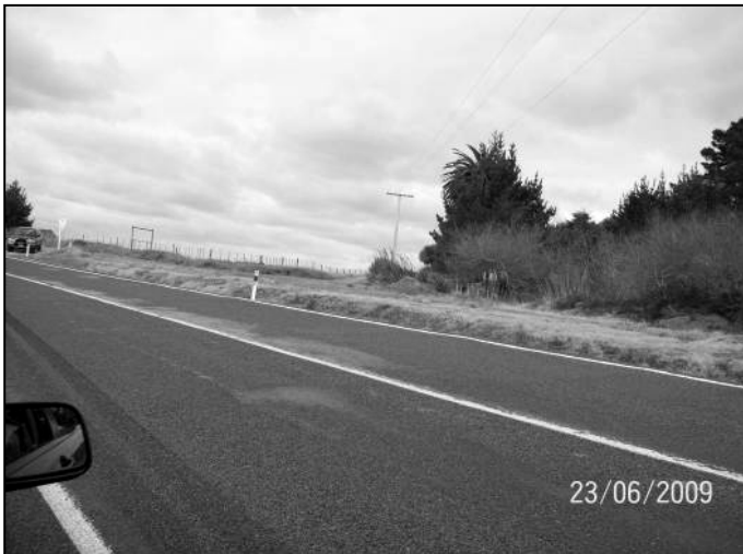
Figure 4.39 View of site C10, showing another area of flushing
