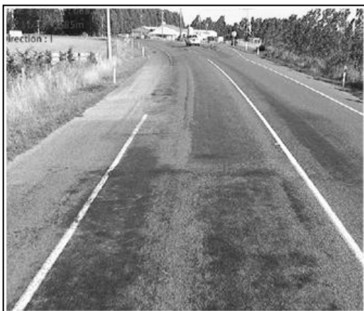
Figure 5.40 Inspection length in site D2 (RP 1145/6583), showing the poor condition of the pavement
