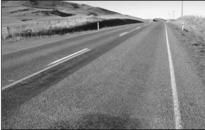
Figure 4.61 View of site D5, showing extensive flushing and rutting
