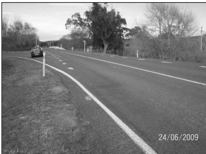
Figure 4.9 View of site B4, showing extensive flushing
