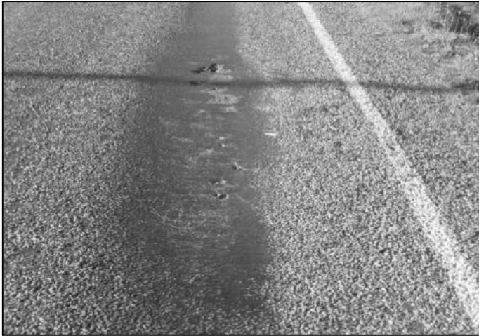
Figure 4.65 View of site D7, showing more detail of the flushing
