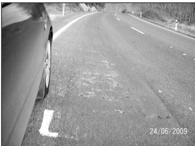
Figure 4.15 View of site B7, showing a failed patchwork repair
