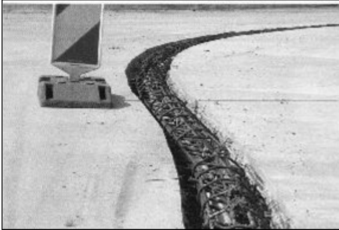
Figure 8.22 In situ construction of the mountable lane dividers: pouring the concrete (CROW 2008)
