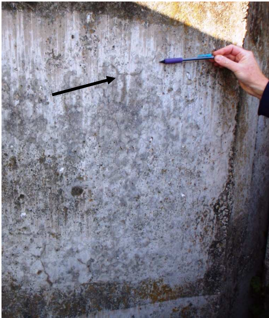
Figure 3.4a Triple point crack (or large-scale craze crack?) on bridge abutment wingwall (Nelson)
