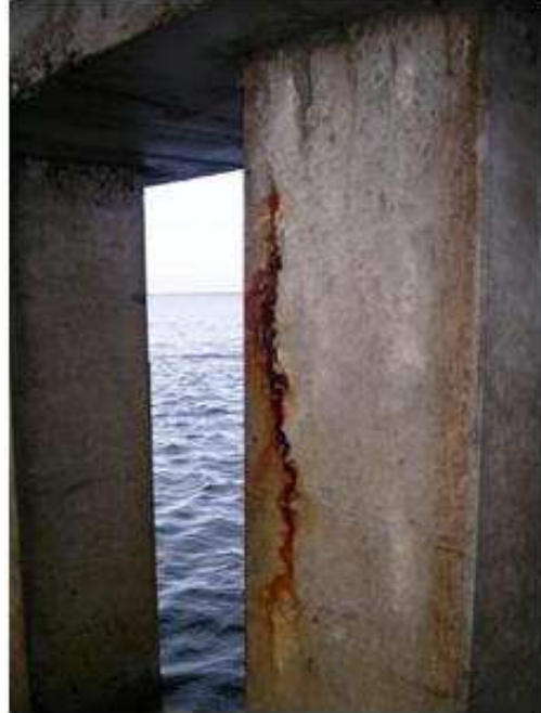
Figure 3.1b Pile cracks caused by reinforcement corrosion (typically wider above high-tide level)
