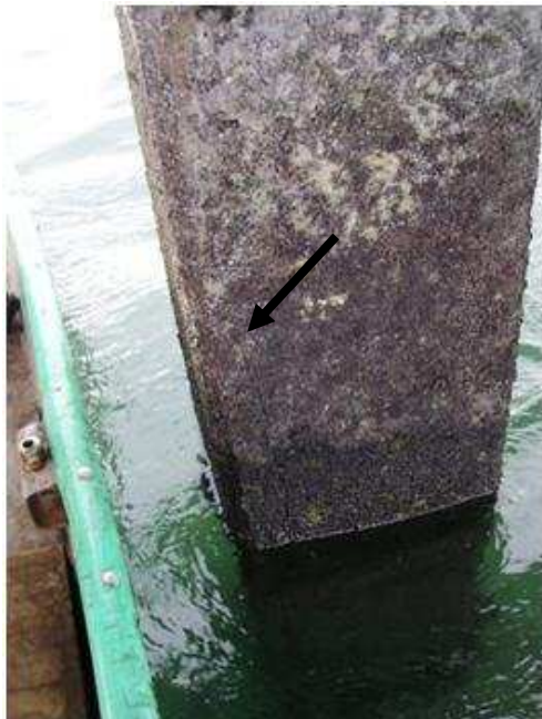
Figure 3.1c Minor ASR/DEF cracking (arrowed)
