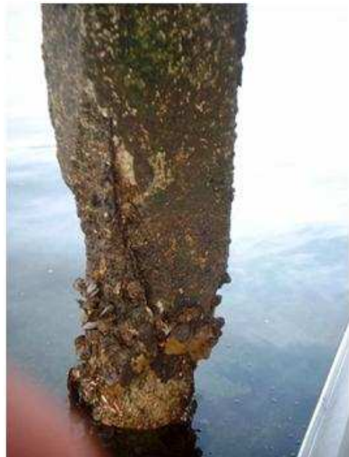
Figure 3.1d Extensive ASR/DEF damage
