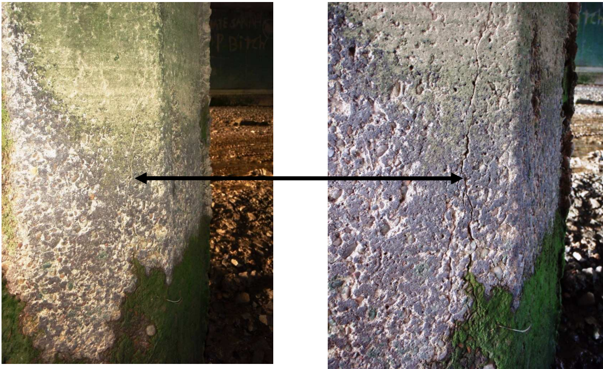
(close-up of crack)
