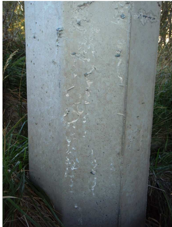
Figure 3.4b Efflorescence on uncracked pile (structure 'O', Southland; see also chapter 4)
