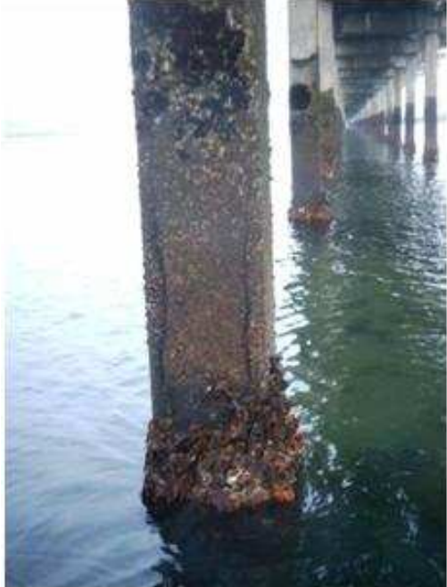
Figure 3.1a Pile cracks caused by ASR/DEF (wider and more common below high-tide level)
