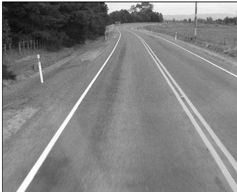
Figure 3.4 The straight section prior to the bridge approach (image from SH53 network video)
