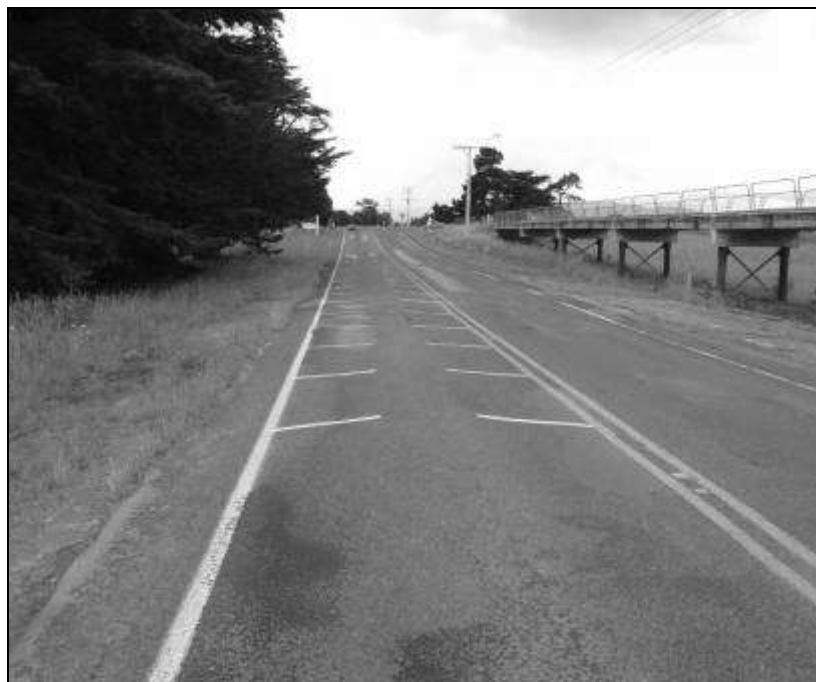
Figure 3.8 Jenkins Dip Floodway bypass on the marked section of the SH53 site.
