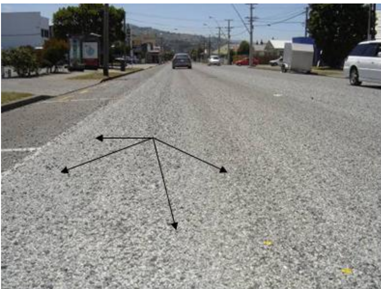
Figure 5.5 Photo showing build up of loose chip on seal surface and on road shoulder
