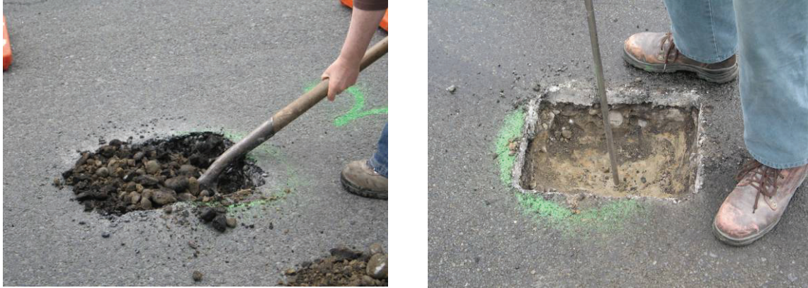
Figure 2.3 Bore hole sampling of Burke St. Removal of seal and construction material (left) and undertaking CBR measurement on exposed subgrade (right)
