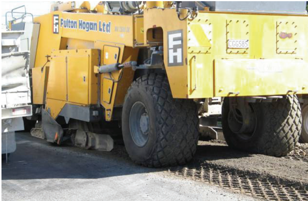
Figure 3.13 Wirtgen 2500 in-situ recycler stabilising Burke St with 3% FB and 1.5% cement – direction of travel is toward the left of the picture, with the stabilised material visible behind the rear wheels of the recycler
