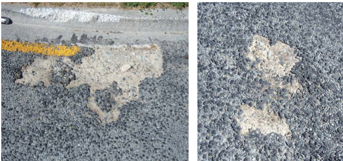
Figure 3.28 Photos (S.McNeill, Christchurch City Council) taken January 2009 (ca nine months after the in-situ pavement recycling) showing chip seal delamination – indicative of weak adhesion between the 'silty' FB-stabilised base and the overlying bituminous chip seal wearing course
