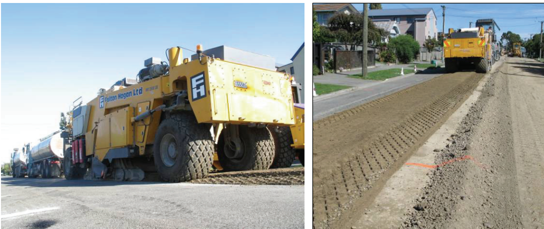
Figure 2.4 Fulton Hogan Wirtgen 2500 recycler – in-situ recycling train consists of recycler, bitumen tanker and water tanker (left). Section of Burke St used for the stabilisation trial and the approximate locations of test section A and B (right)
