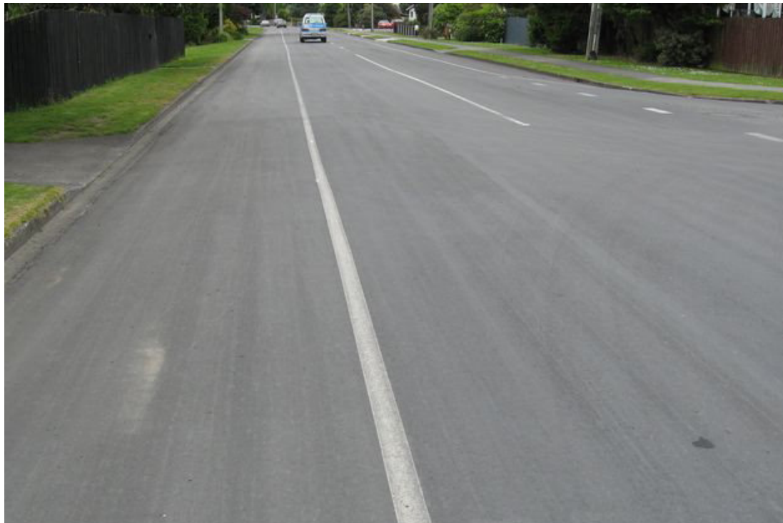
Figure F4 HIGH Q_o . Site 49 Kapiti Coast: A light asphaltic concrete surface with Q_o 0.084 , ( S1 = 0.53 ). Lighting this surface effectively would require only a small fraction (as little as 1/3) of the energy required to light the surface shown in figure F_3.
