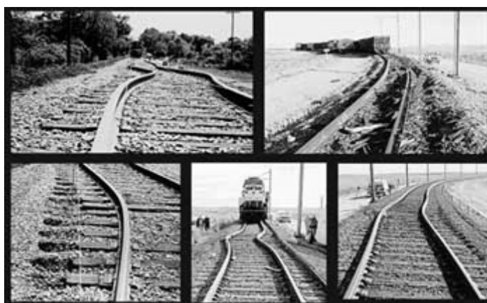
Figure 3.1 Track buckle illustrations (Source: Volpe National Transportation Systems Center 2008).
