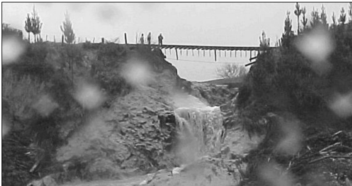
Figure 5.2 Washout caused by flooding affects the national rail network (location unknown).
