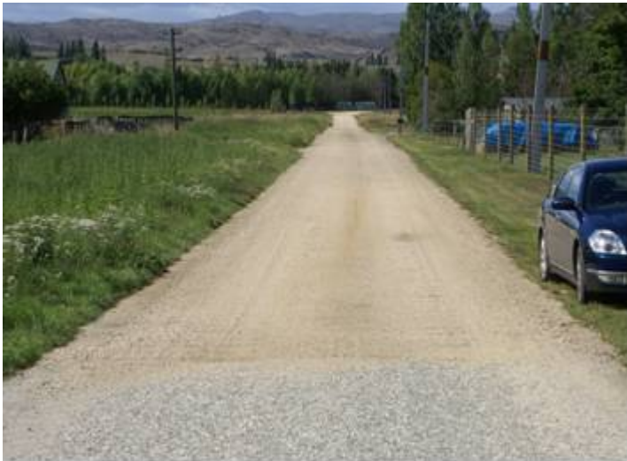
Figure A1.6 Keddell Road - from end of Otta seal, looking south at oil section
