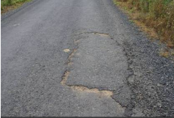
Figure 6.3 Surface shear failure, Church Road site (Jan 2008)
