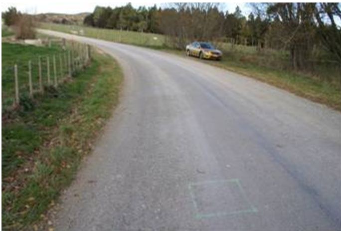
Figure A1.11 Paroa Road - Otta seal, looking south to start of emulsion section
