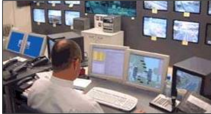
Figure 2.8 ATTOMS Control Centre.
