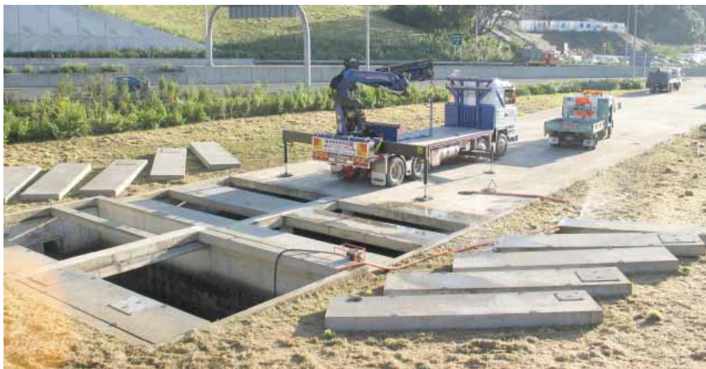
Figure 2.4 The 100 m long Grafton Gully SWTD, showing the fully uncovered inlet chamber (first compartment to the left) and the partially uncovered forebay chamber (in between the inlet and the Hiab truck).
