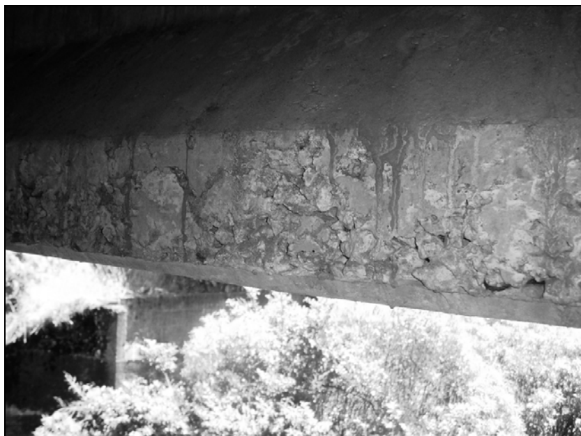
Figure 5.6 Poor compaction on beam, Sandy's Bridge.
