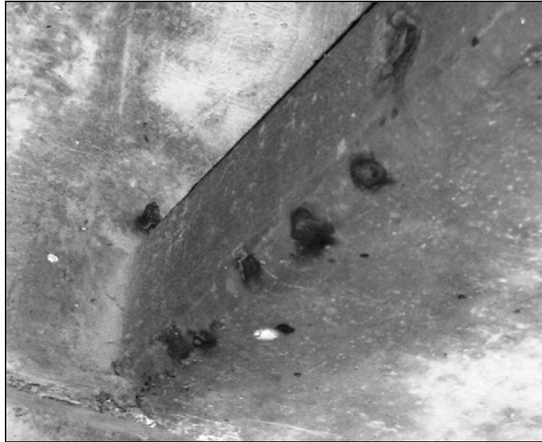
Figure 5.5 Corroding stirrup ends close to surface on Hawai River Bridge.
