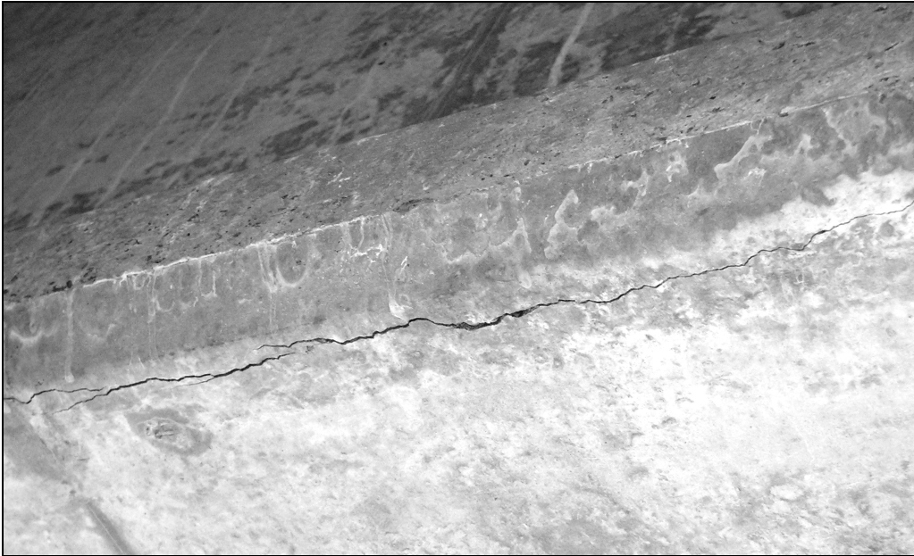
Figure 5.2 Cracking over a prestressing strand on the Hamanatua Stream Bridge.
