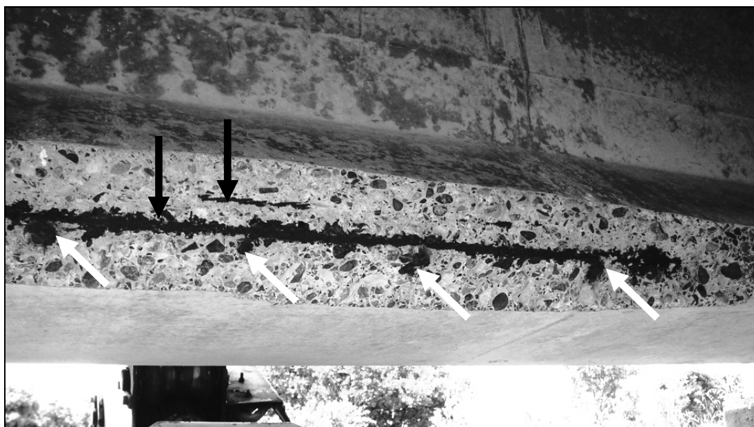
Figure 5.1 Spalling over prestressing strand on the Hamanatua Stream Bridge, Span BC.
