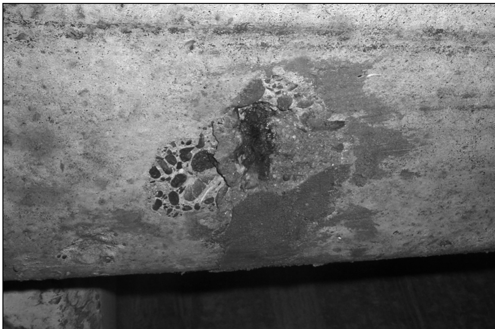
Figure 5.4 Spalling associated with low cover over a stirrup on the beam soffit, Kereu Bridge.
