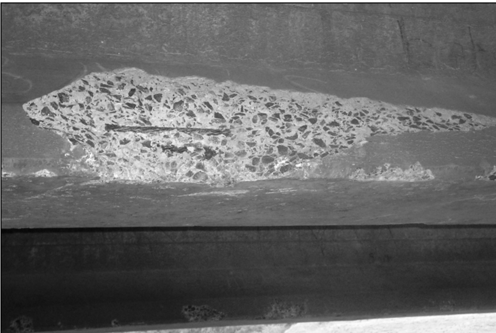
Figure 5.3 Corroding strand on Hawai River Bridge. This spall was caused by impact damage rather than corrosion.
