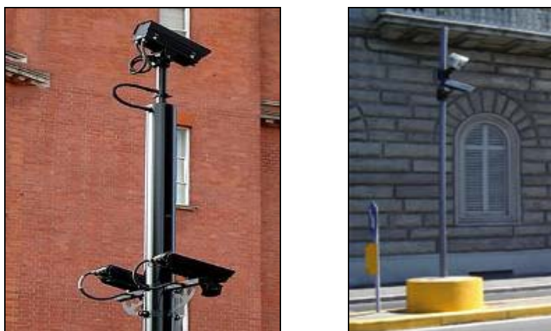
Figure 4.14 Typical camera installations.
