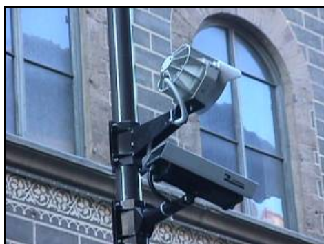
Typical ANPR camera & illumination device.
