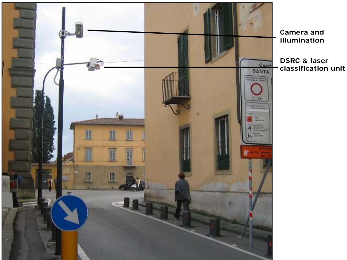
Figure 4.5 Typical street based DSRC installation.
