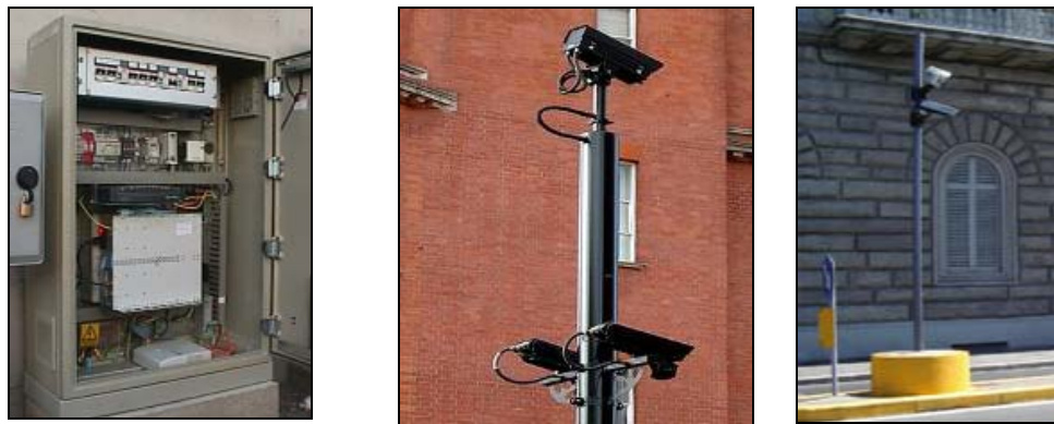
Typical cabinet. Typical camera installations Figure 4.3 ANPR cabinet and camera installations.
