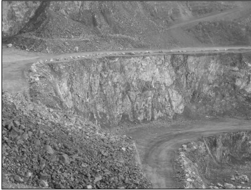
Figure A5 Drury greywacke quarry, showing how the rock is strongly jointed and fractured.
