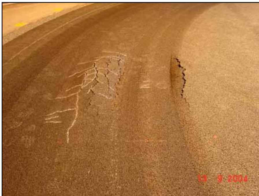
Figure 2.7 Failure between Stations 25-27 at 0 load cycles.
