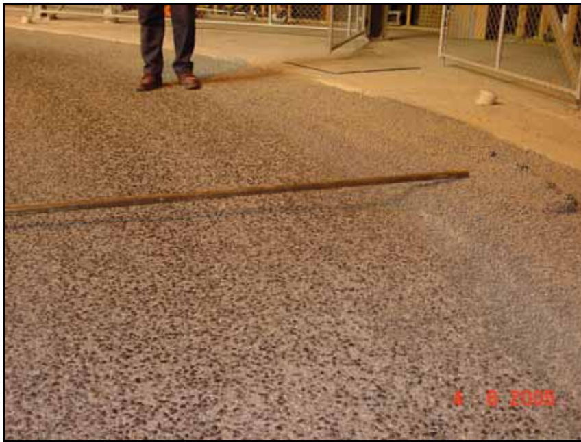
Figure 4.4 Initial construction shear failure between Stations 20–24.
