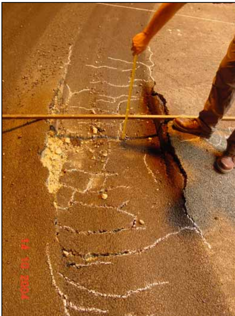
Figure 2.9 Failure between Stations 29–33 at 120,000 ESA.
