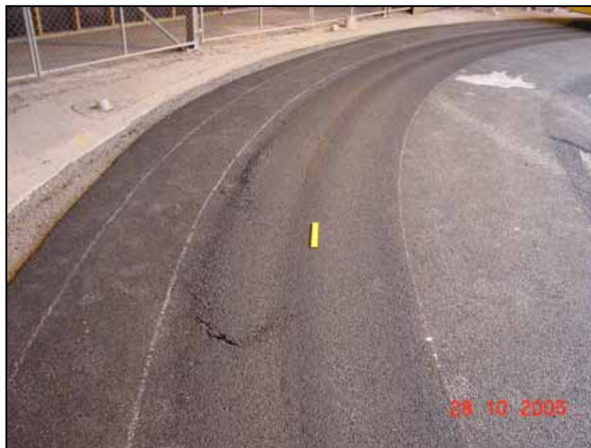
Figure 4.7 OGPA debonding failure at 200,000 ESA between Stations 25–27.
