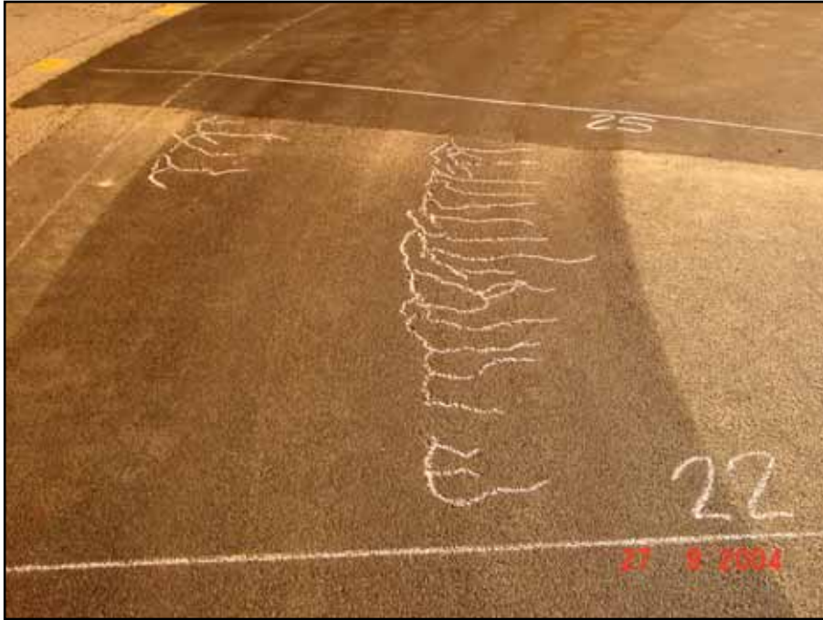
Figure 2.8 Failure at Stations 22–24 at 36,000 ESA.
