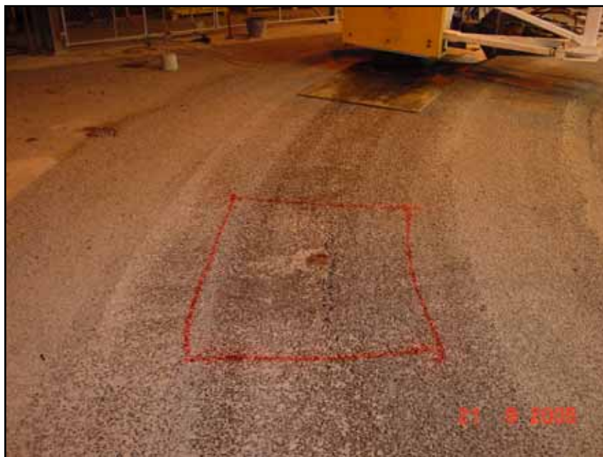
Figure 4.5 Typical surface failures that occurred at different stations during Pavement Test 2.
