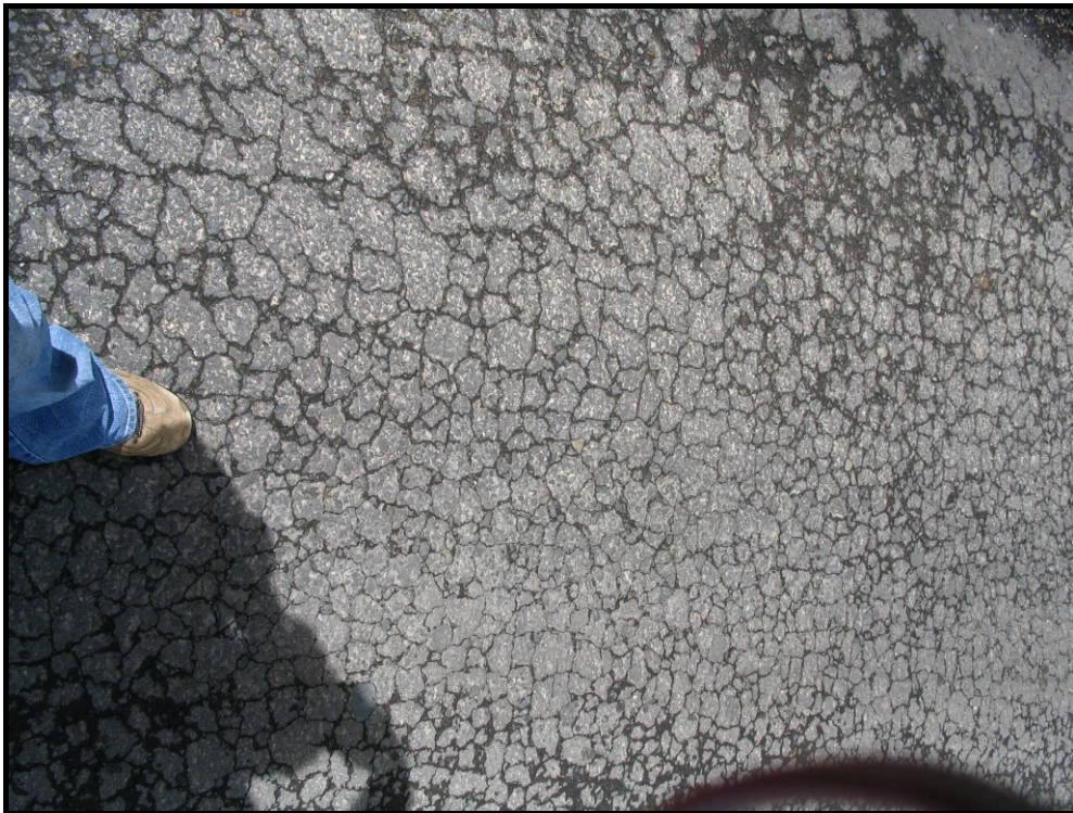
Figure 4.7 Detailed view of crocodile-cracked surface.
