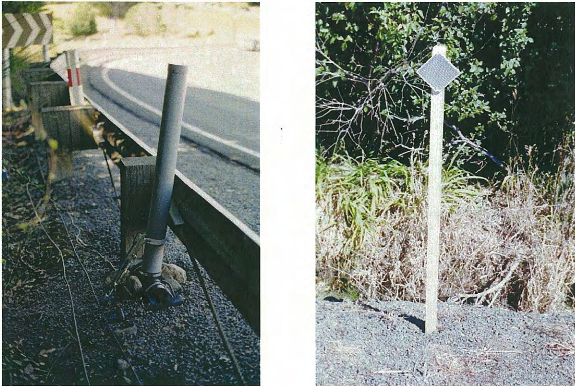
Figure 3.2 Typical optical sensor and reflector.
